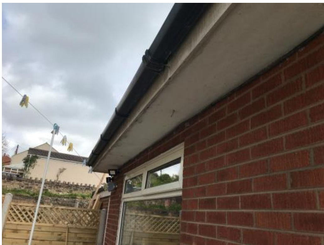
Plate 4 – Tightly sealed soffit box on the rear elevation
