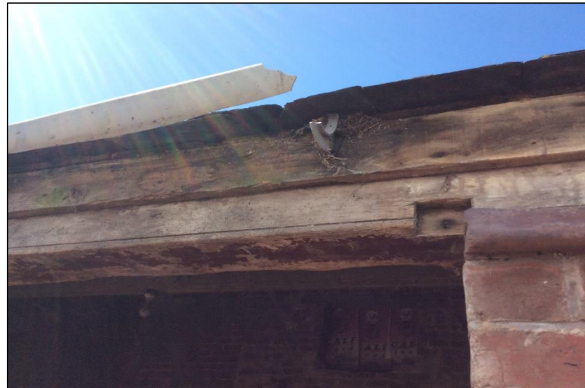
Gaps under the tiles on the eastern elevation.
