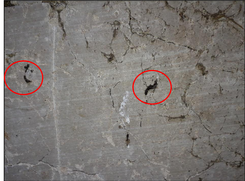
Droppings on the wall, located centrally.
