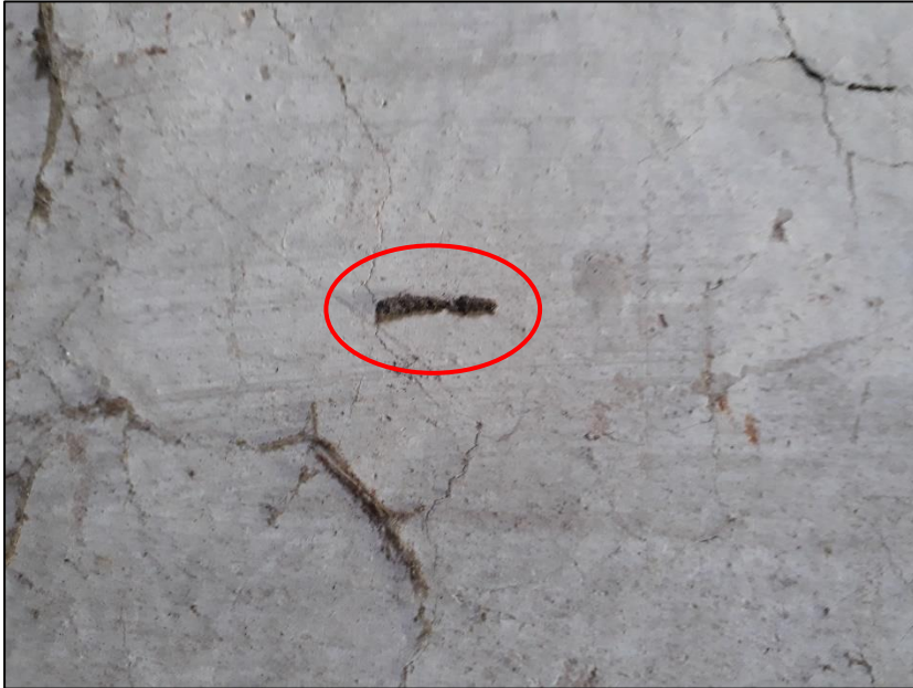
Droppings on the wall, located centrally.
