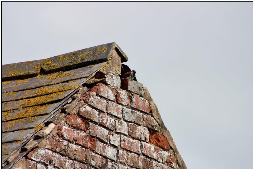
Gaps in the brickwork and missing mortar on the southern gable end.
