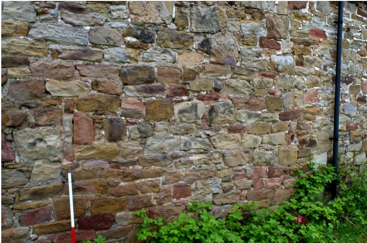
Figure 38 West elevation West Range Blocked ventilator slits at lower level
