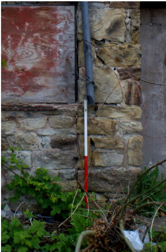
Figure 30 Straight joint below lean-to window
