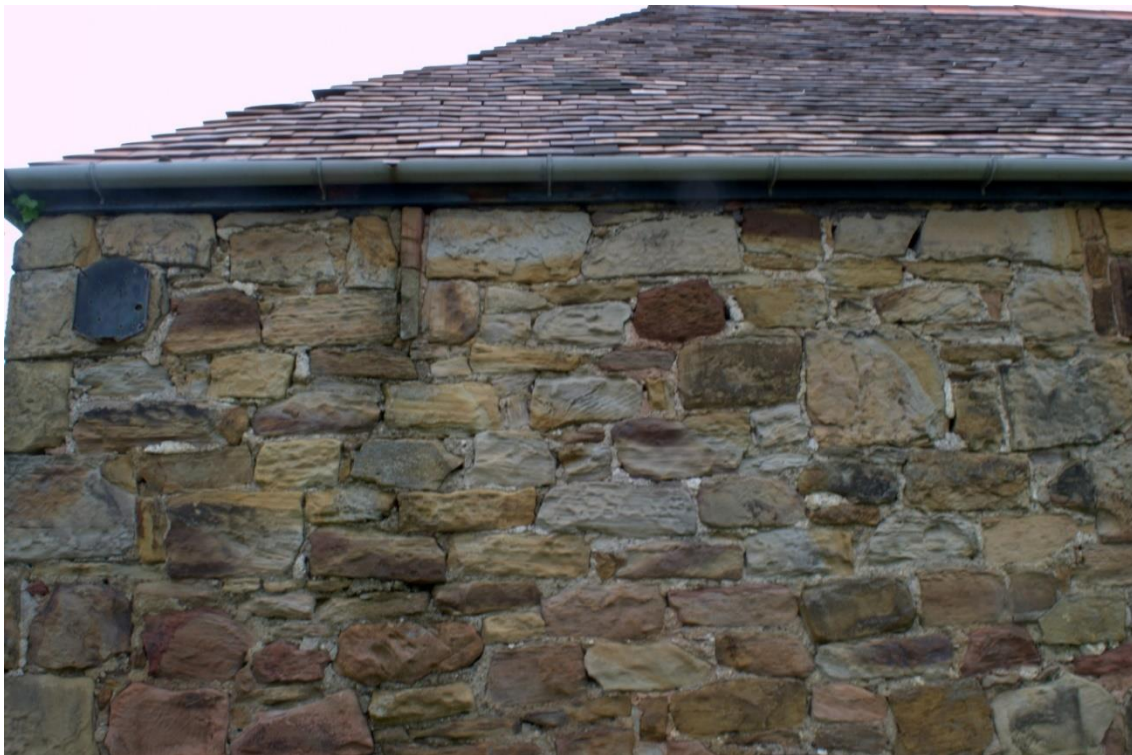
Figure 37 West elevation West Range Blocked ventilator slits below eaves
