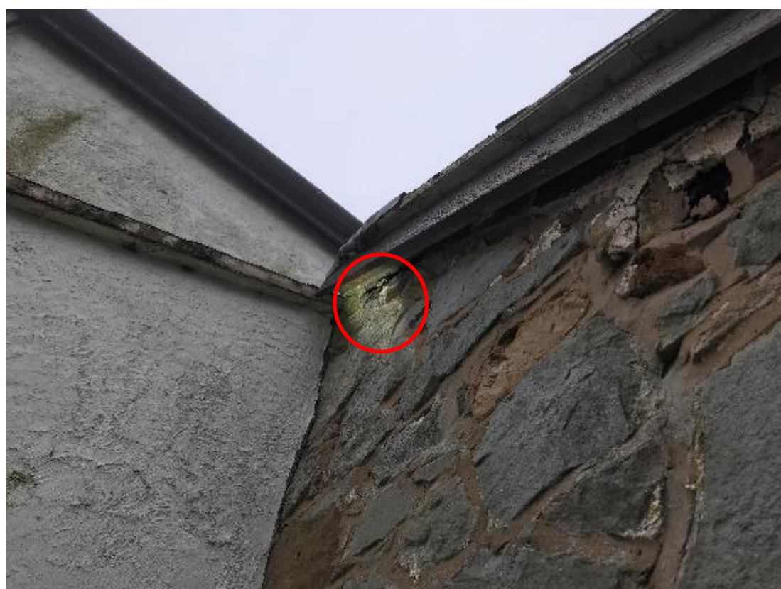
Plate 6 – Gap behind the fascia of the original dwelling in proximity to the extension
