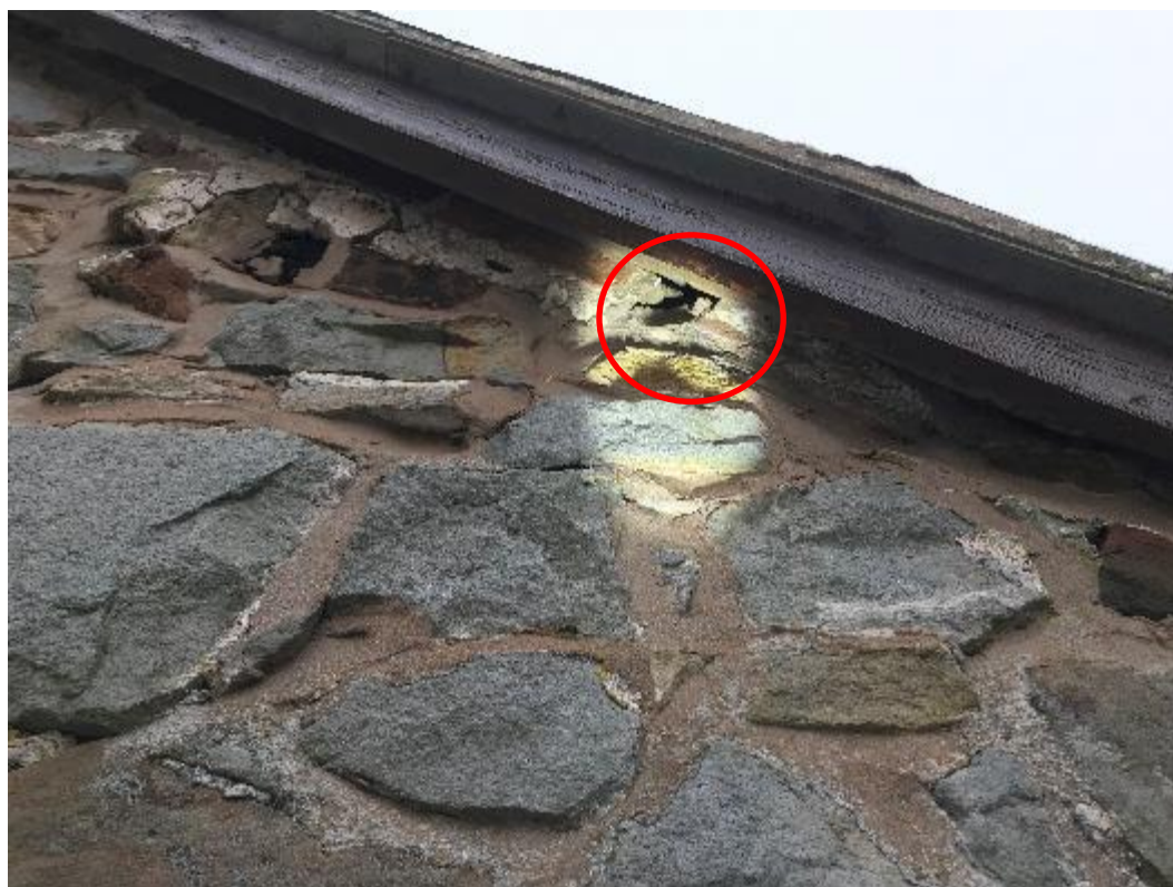
Plate 5 – Gap behind the fascia of the original dwelling
