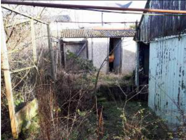
12.01.18 – Shed located along centre of western boundary; suspected asbestos cement sheet cladding and roof.
