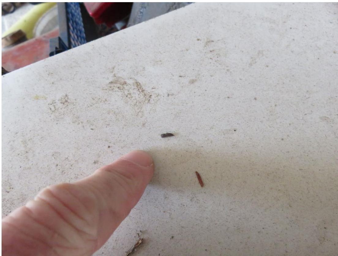
Photograph 13 – Single bat dropping found in larger ground floor room
