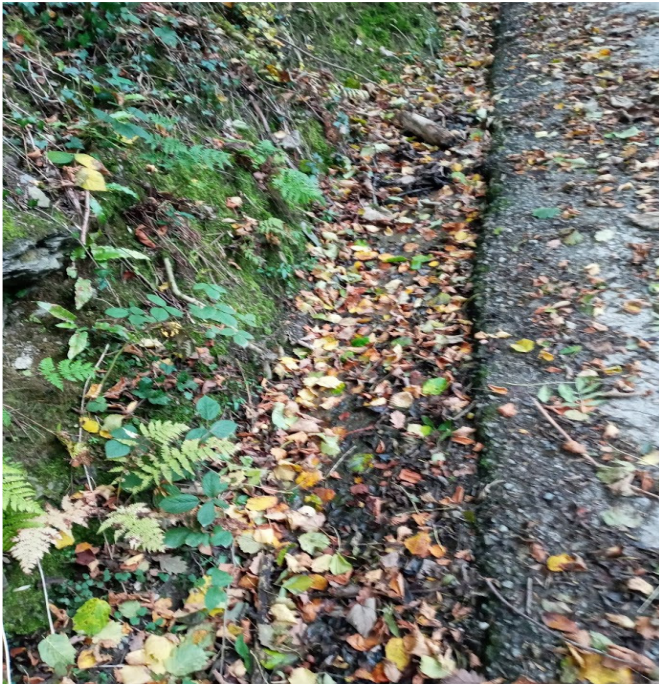
Channel formed by water erosion at LH side of road
