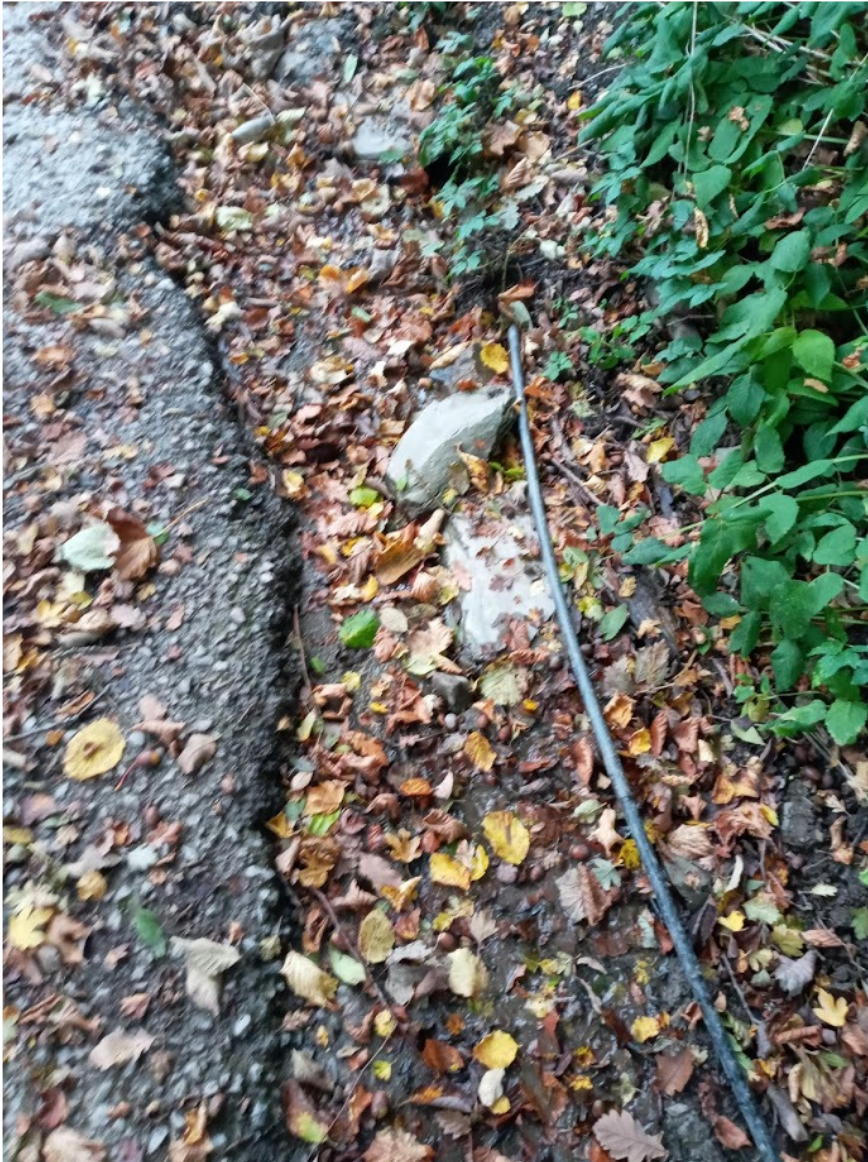
Channel formed by water erosion at RH side of road
