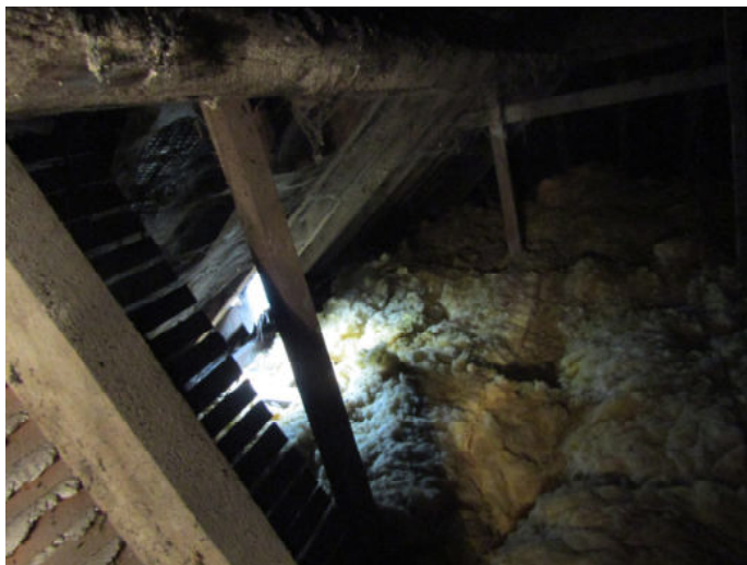
Photo 3: Missing slates create a hole, which provides a 'fly-in' access in the roof.
