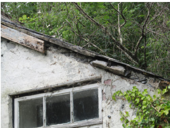
Photo 6: Gaps under eaves provide potential bat access.
