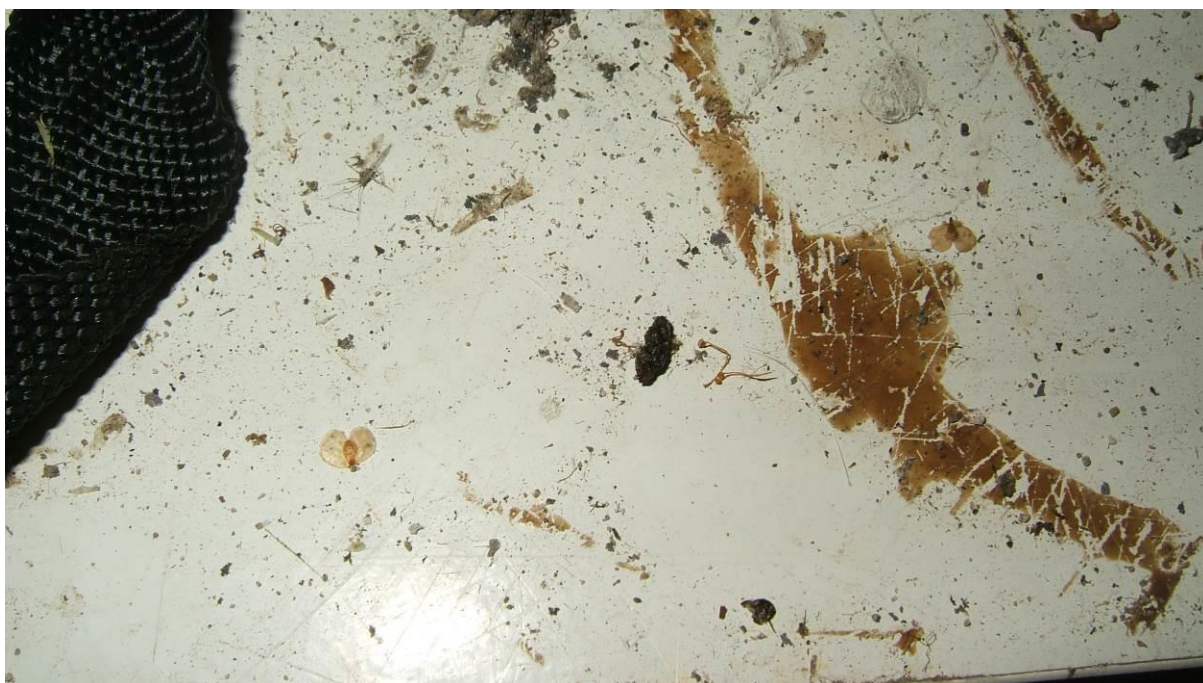
Figure 9: Bat dropping inside Building 3.
