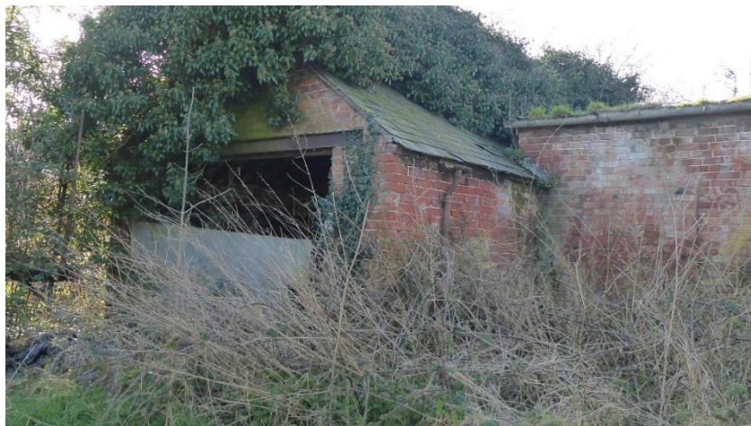
Figure 4.22 Gaps between tiles
