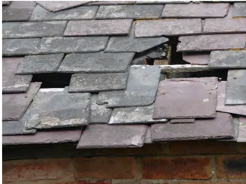
The holes in the roof of the building at Target Note 4b.
