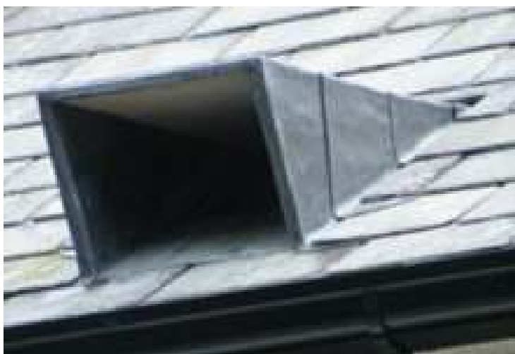
Figure 4: possible access point into bat loft
