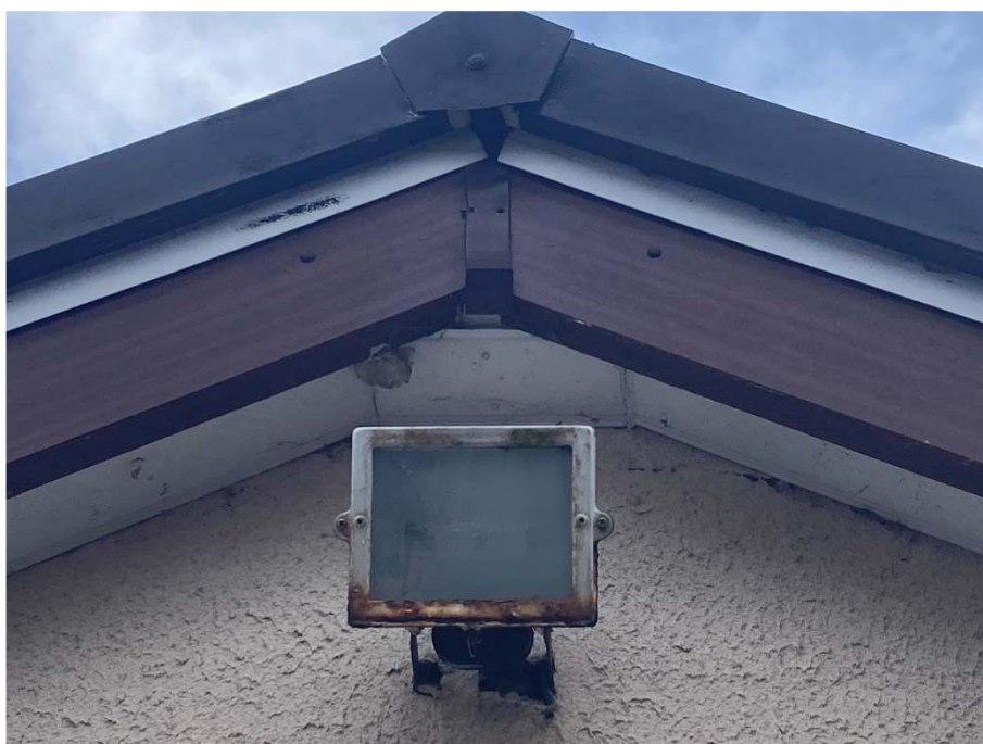
A1.8 Plate 8: Gap beneath cap of barge board on western aspect (front)
