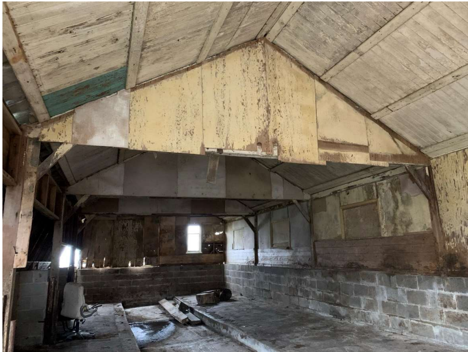
Photograph 5; patchwork of timber boards on the western elevation
