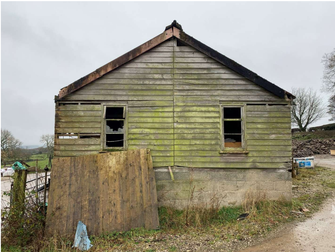
Photograph 3; northern gable showing metal barge boards – heavily rusted
