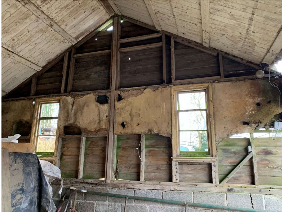
Photograph 4; patched and rotting boards on northern gable
