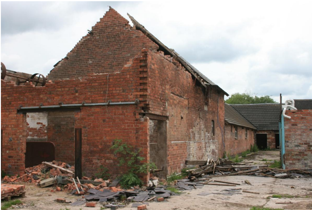
The 'L-shaped barn' looking east. Before its collapse, the ruined gable had probably had the neoclassical detailing in engineering brick exhibited by all the 'estate phase' buildings
