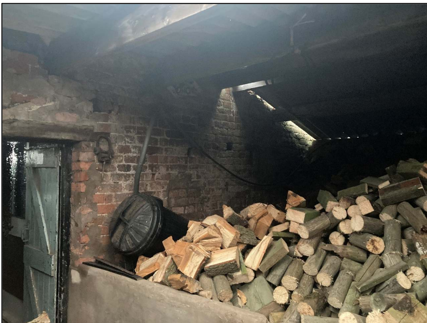
A1.10 Plate 10: Example of interior gaps between brickwork
