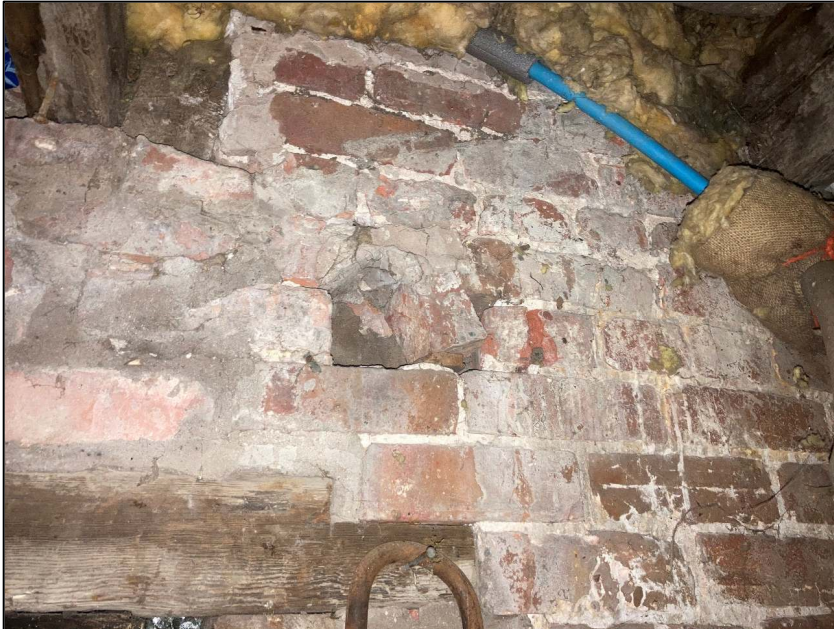
A1.9 Plate 9: Interior of section 3 with gaps in brickwork
