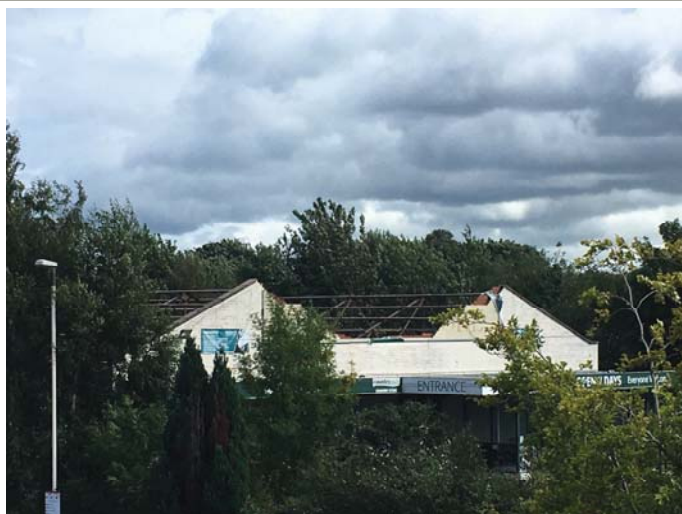
Photograph 7 – Building P2-B1 showing missing roof and broken wall
