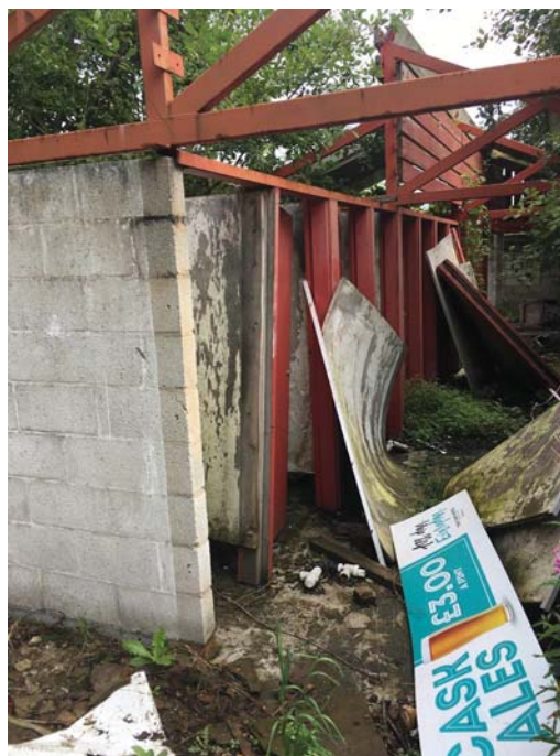
Photograph 6 – Interior of Building P1-B2 showing missing roof and dilapidated condition
