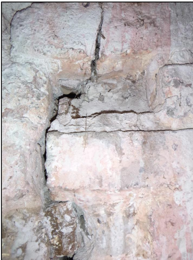
Photograph 3 showing crack in internal wall
