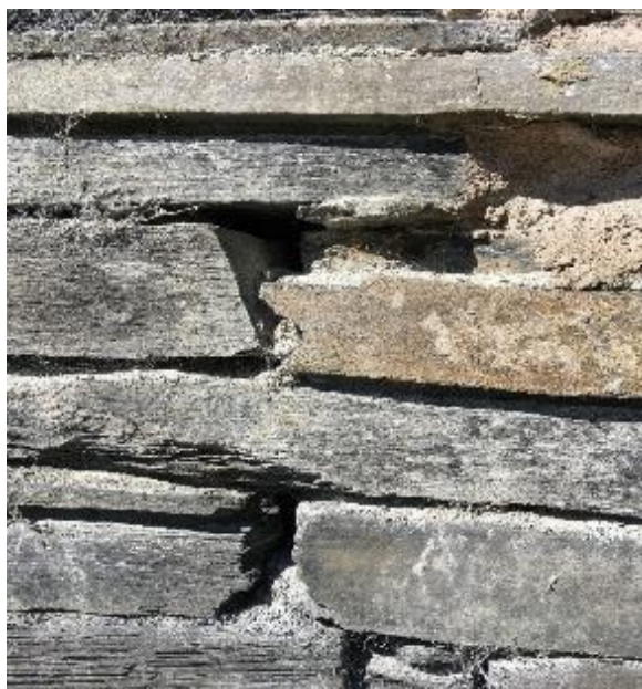
PR8 Gaps in stonework
