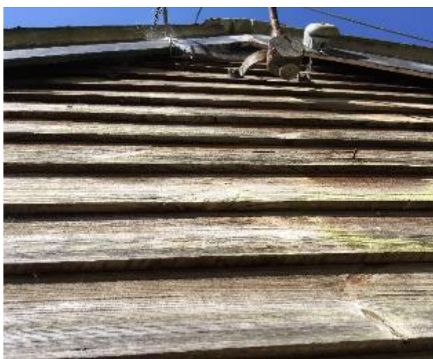
PR6: Gap under fascia boarding, the weather boarding has no backing, so no cavity
