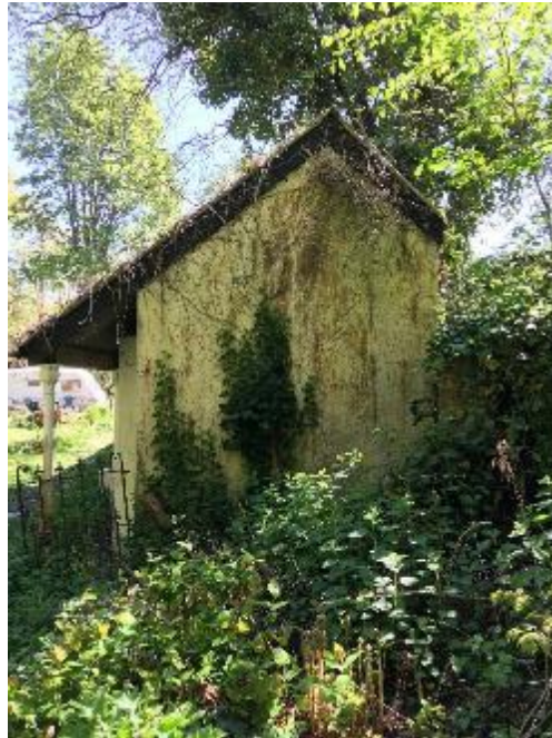
PR2: West gable end, no potential under fascia boarding here, damp and cool, fascia boarding close fitting.
