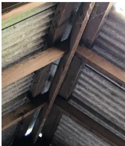
PR9: Internal roof structure, gaps under ridge into building
