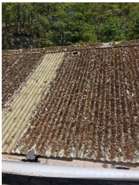
PR7 Gap in asbestos roof – south elevation
