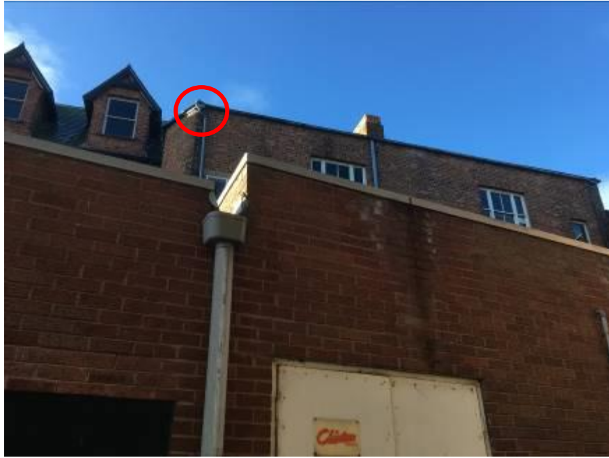
Plate 6: Minor damage on the north-east corner of the building at the roof verge
