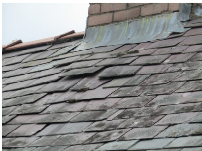
Photo 3: A few gaps were observed beneath slates and ridge tiles.
