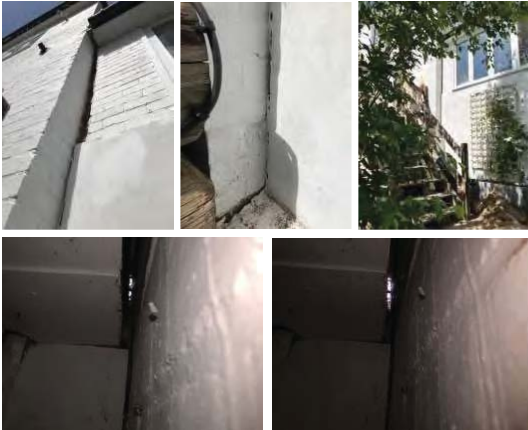
Figure 6 - Vertical gaps / cracking at extension interaction with historic structure
