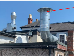
Modified Existing Stainless Steel Flue Approx Height 1200m above roof line
