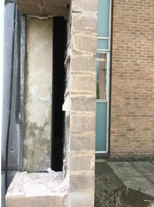
Plate 5: Major gap leading to wall cavity on western end of North face
