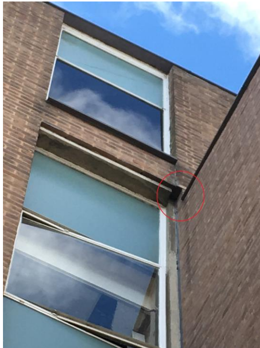
Plate 4: Minor gap above sash window in North-West inside corner
