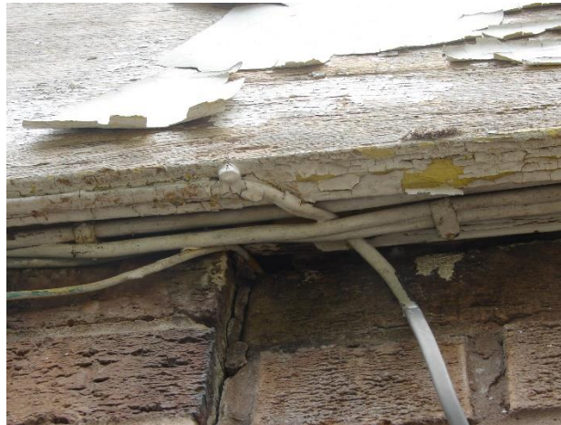
Photo 4.8: Small gap beneath fascia on single-storey section
