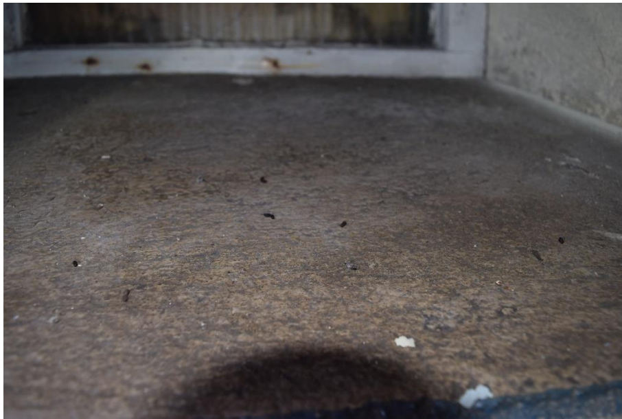
Figure 4.6. Droppings on window ledges
