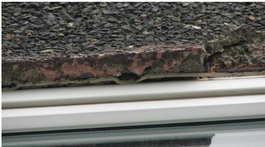
Minor gap above a window on the western elevation.
