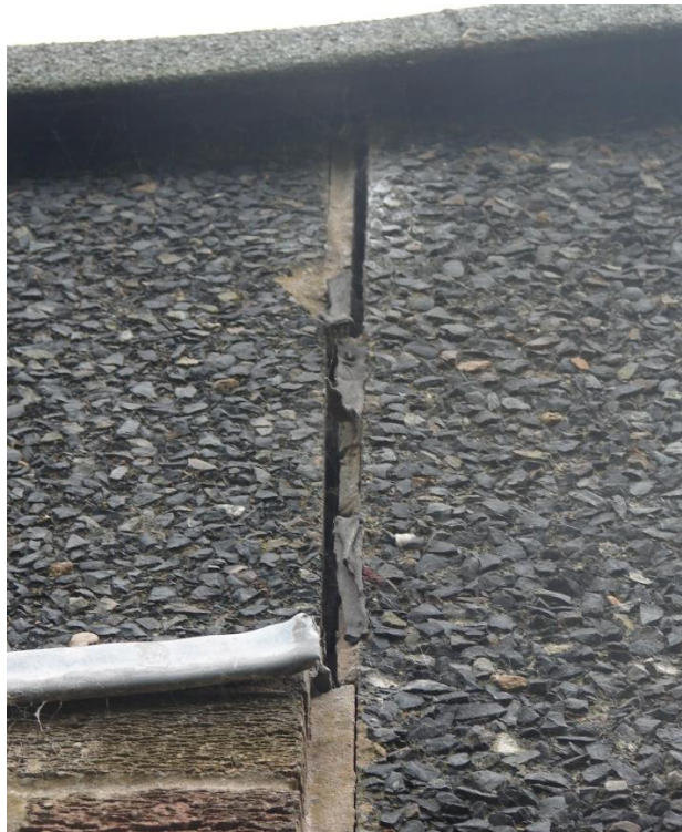
One of the gaps between concrete panels on the northern elevation.
