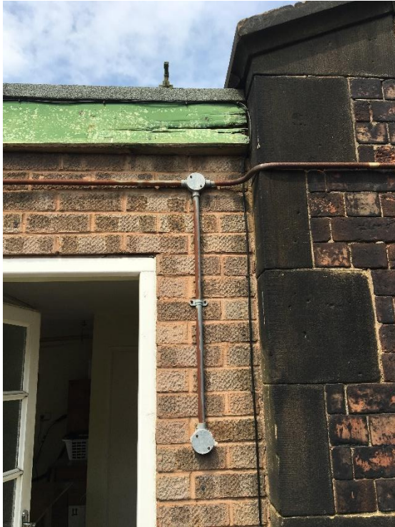
Warped fascia board painted green on east elevation
