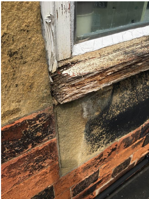
Rotting timber on the window frames to the extension and to the kitchen
