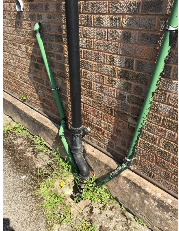
Green pipework to south elevation
