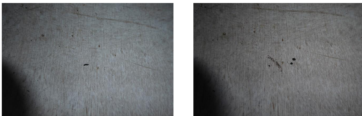
Figure 4.16. Bat droppings in loft
