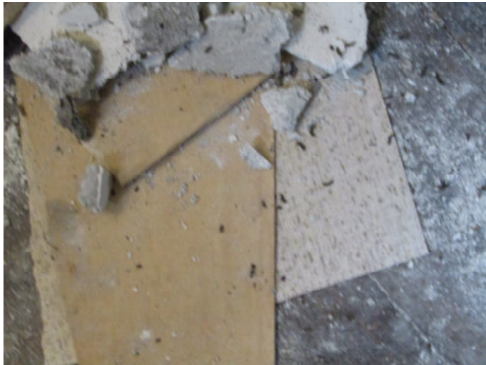
Photo 1: Bat droppings on bathroom floor.
