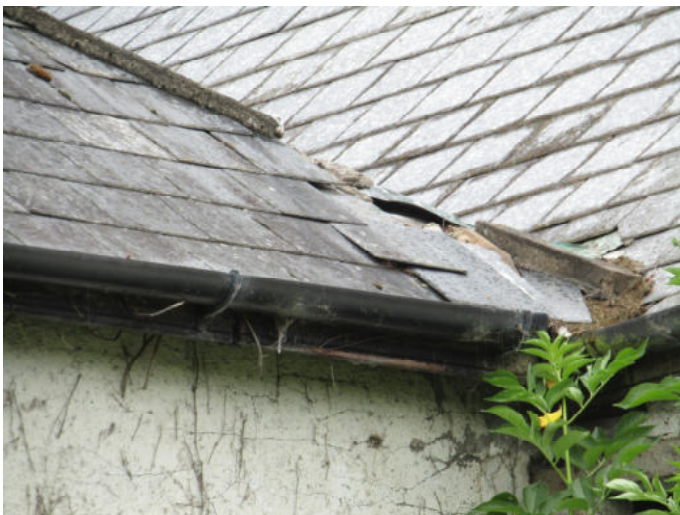
Photo 5: Gaps beneath slates provide potential bat access.
