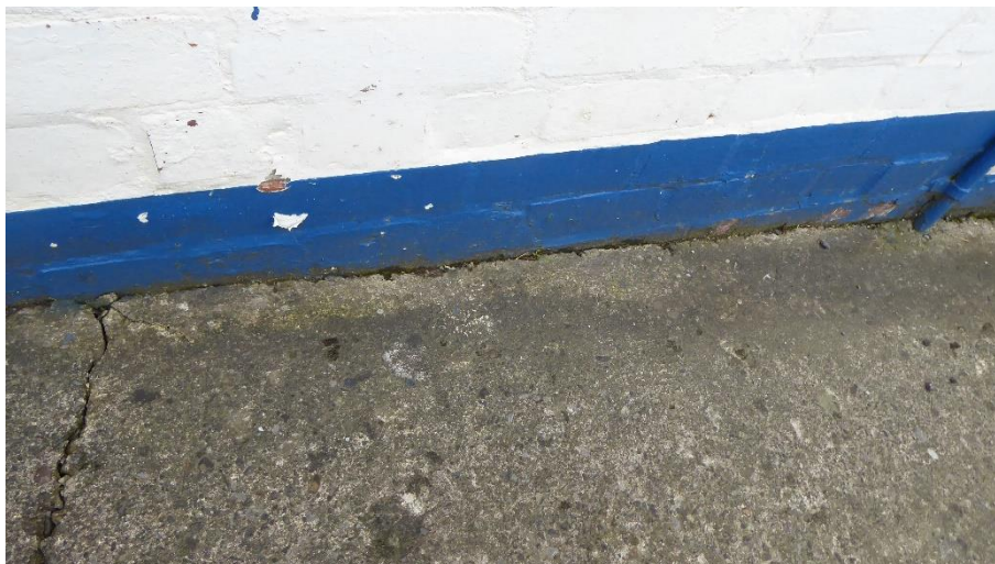
Figure 4.14. No suitable gap around the base of the buildings
