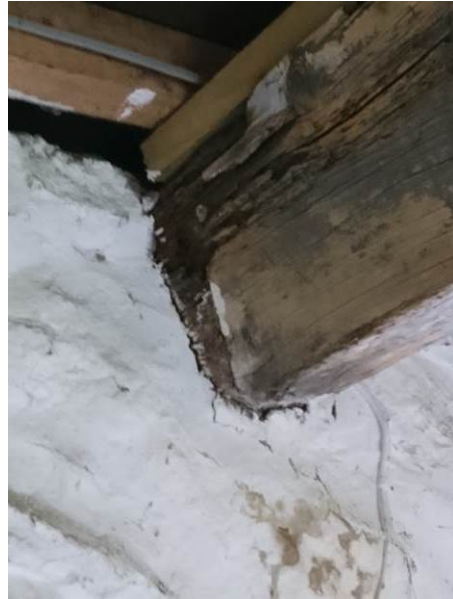
Slight rot at purlin end.
