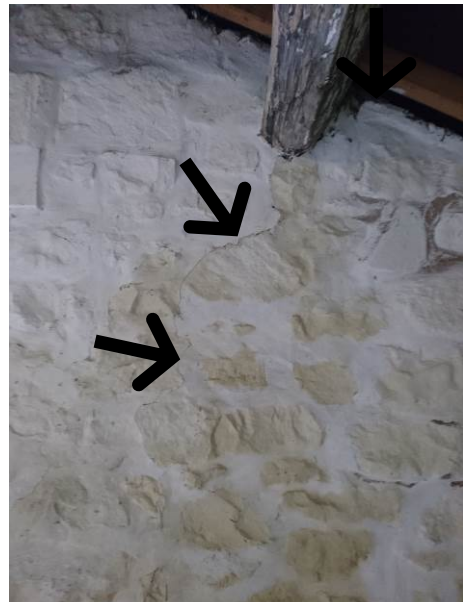
Cracking extending down from purlin bearing.
