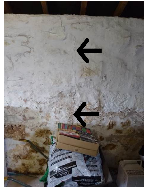
Damp staining at low level. Vertical crack to left hand side elevation.
