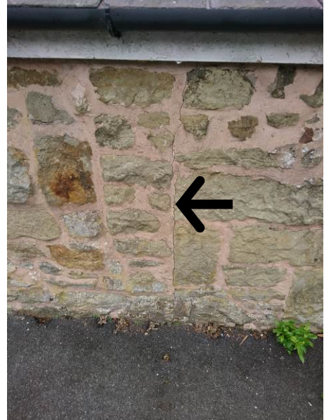
Vertical crack to left hand side elevation.
