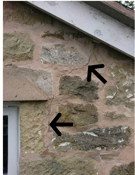
Cracking adjacent to window on rear elevation.
