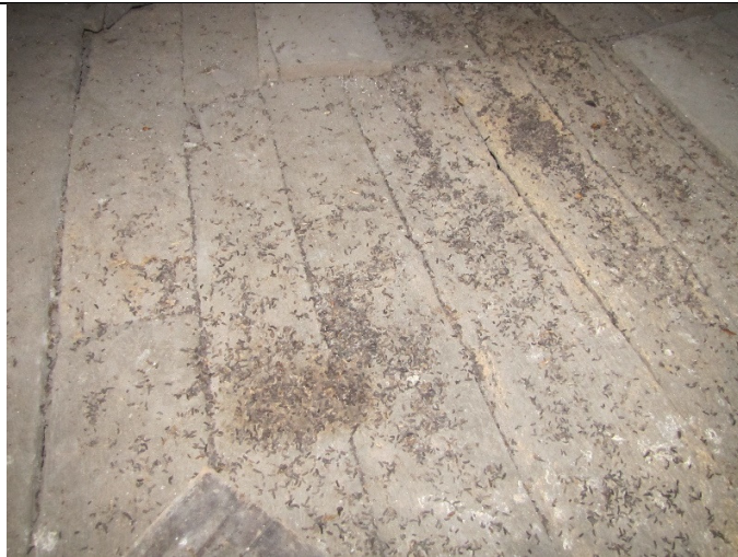
ABUNDANT BAT DROPPINGS ON LOFT FLOOR BUILDING 3
