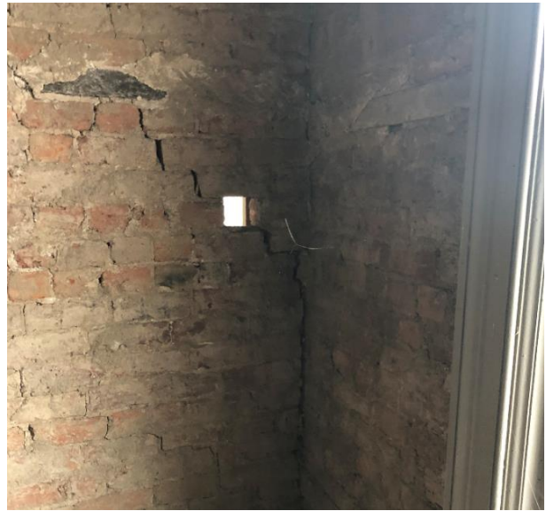
Fig 4: Stepped cracking and vertical crack along interface with front elevation suggesting restraint to front elevation has been severed
