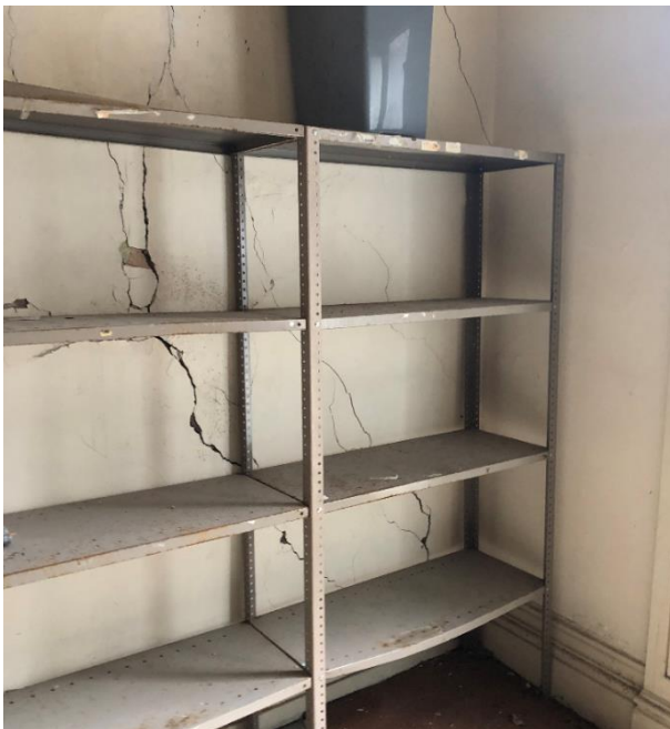
Fig 1: Settlement cracks to internal wall adjacent to front elevation
