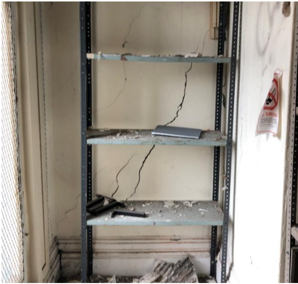
Fig 3: tapered cracking adjacent to front elevation – significant settlement of central portion of masonry leading to severe cracking to return walls
