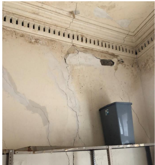
Fig 2: cracking extending full height to ceilings
