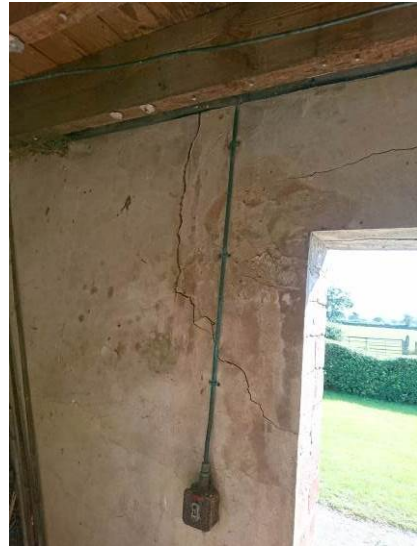
Photo 15 – Cracking to side of door opening.
