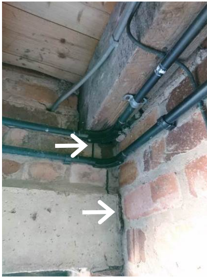
Photo 17 – Cracking to side of door opening.
