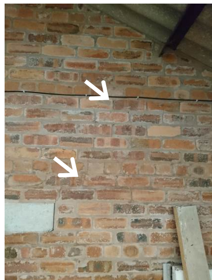
Photo 11 – Cracking to front elevation.
