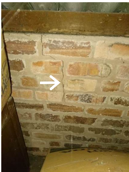
Photo 13 – cracking to right hand side elevation.
