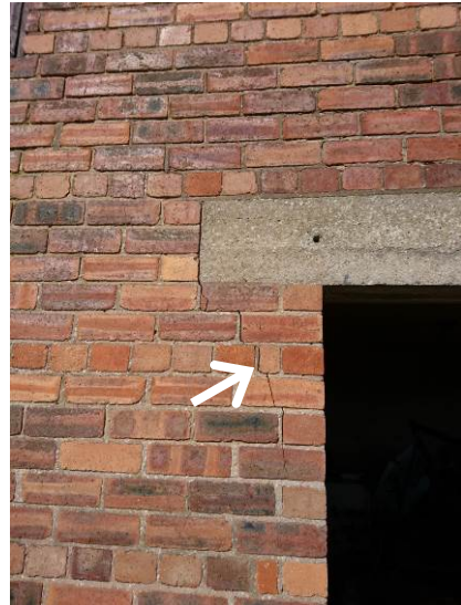
Photo 3 – Cracking below lintel.
