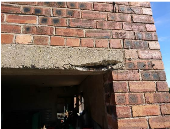
Photo 7 – Spall to concrete lintel.
