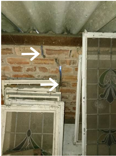
Photo 12 – cracking to left hand side elevation.
