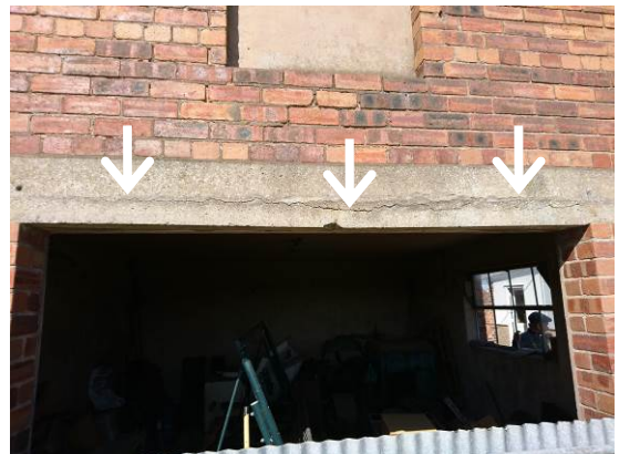
Photo 4 – Cracking to concrete lintel.
