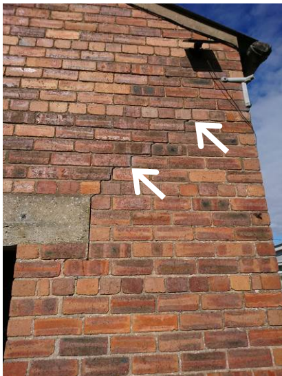
Photo 2 – Cracking to right of door opening.
