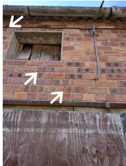
Photos 9 – Cracking above door opening.
