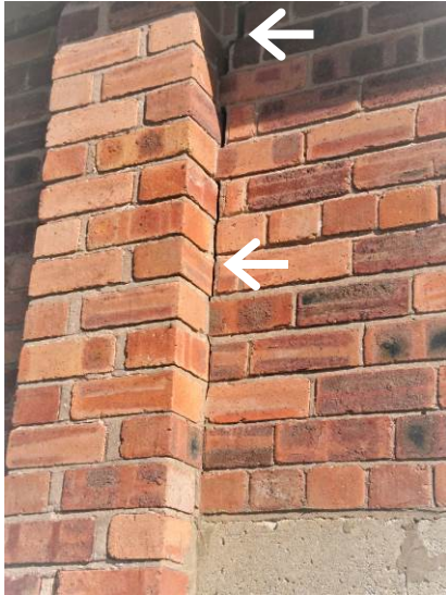
Photo 6 – Cracking extending from door opening.
