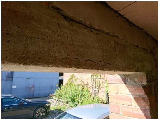
Photo 14 – cracking to door lintel.
