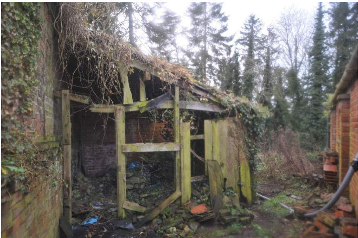
Pl.47: Derelict timber shed at west end of the complex.
