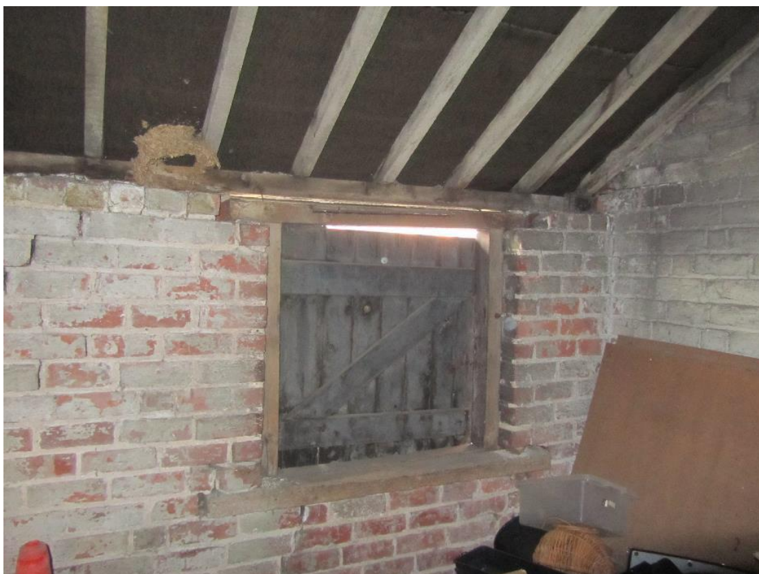
Image 3.30 Gap above a shutter on the first-floor level of B3 presenting a potential access opportunity
