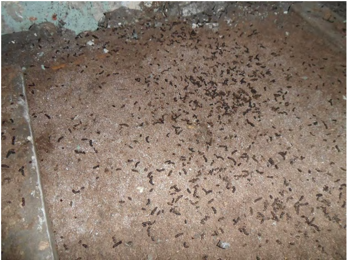
15. Droppings on top of the loft hatch beneath the ridge beam on the south west side of the building.
