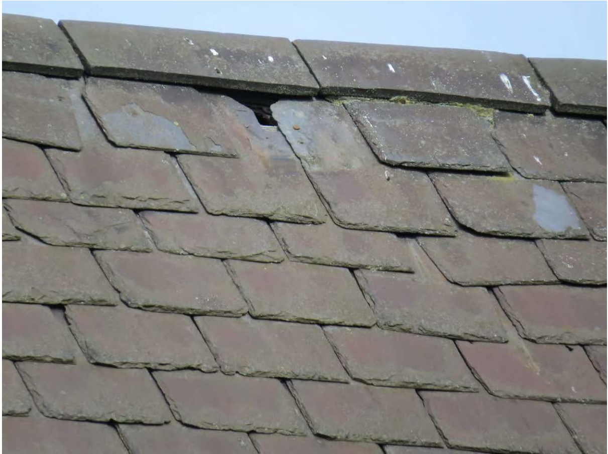
5. There are gaps between roof and ridge tiles which could be used by roosting bats.
