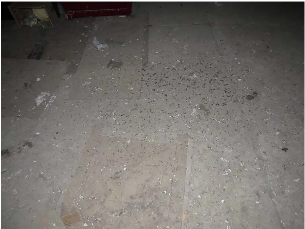
14. An accumulation of droppings beneath a hole in the plasterwork of the roof space above.
