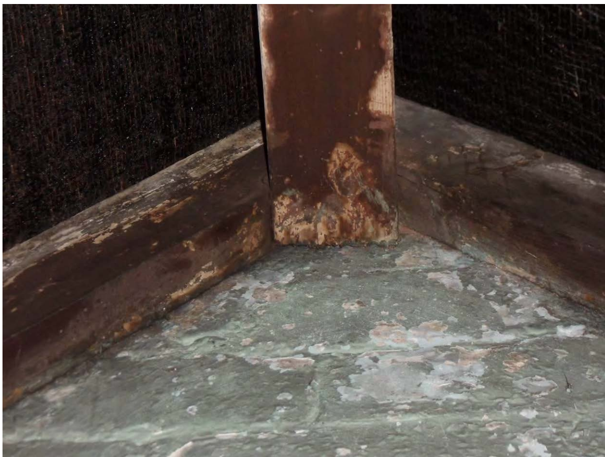
18. Wear marks on the ridge beam at above the loft hatch on the south west gable end.
