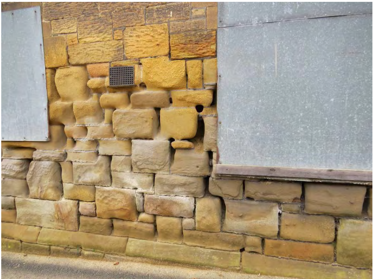
4. The stonework has eroded leaving numerous gaps between blocks.
