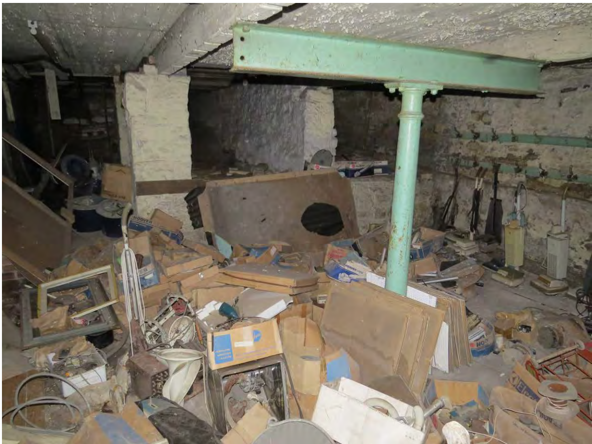
10. There is a cellar beneath the central section of the building, scattered bat droppings were found.
