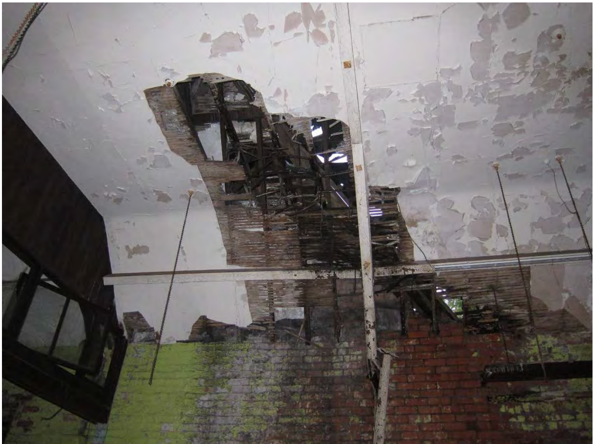
6. The hole in the roof of the central section where bats were seen to enter / exit.
