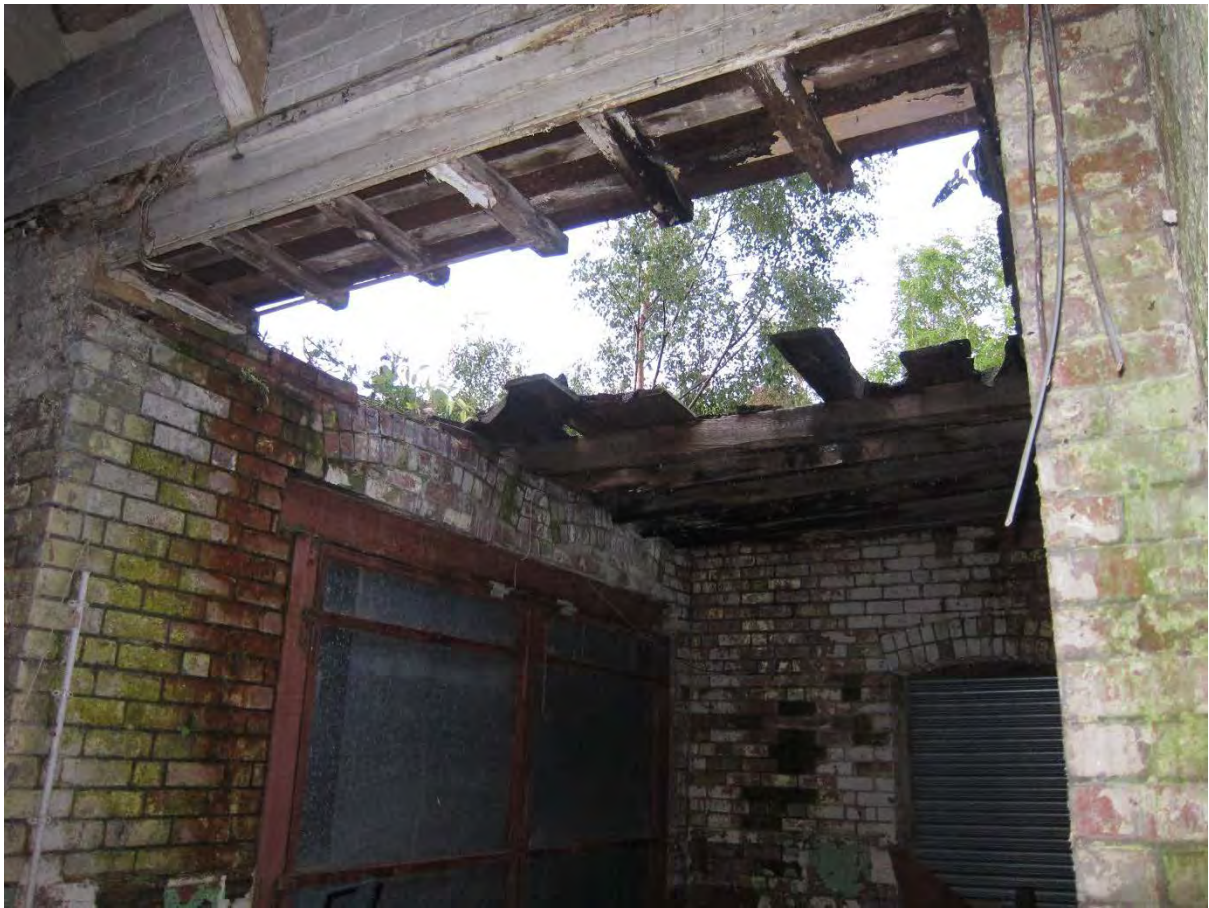
7. The hole in the flat roof section (north) where bats were seen to enter / exit.
