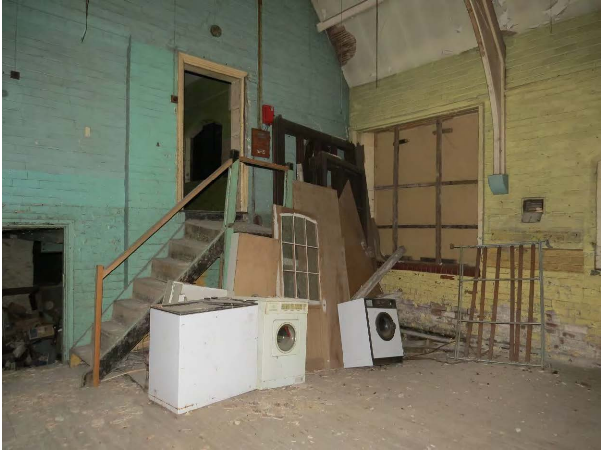
9. The floor is collapsing in some sections of the building, here in the northern section.
