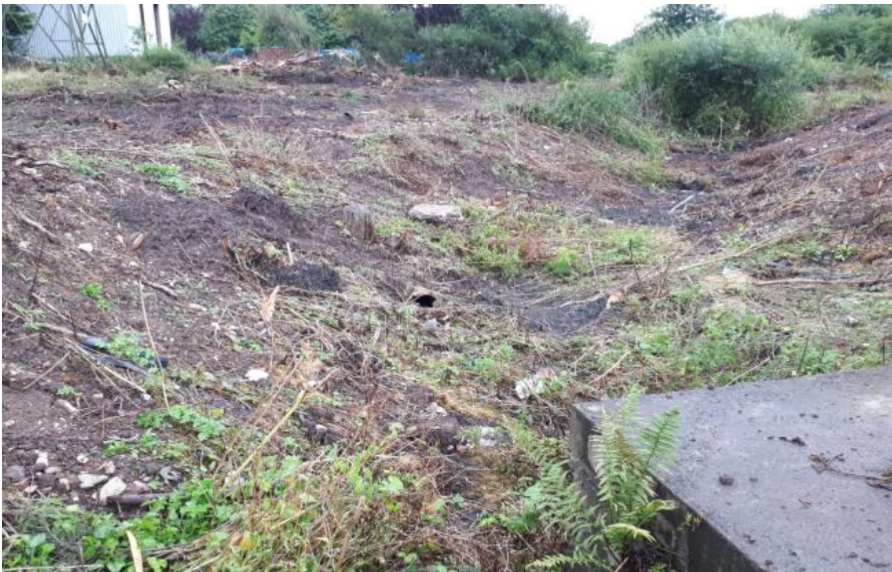
Photo 5: View East: Gully leading from concrete service cover. Drainage pipe exposed in northern gully face
