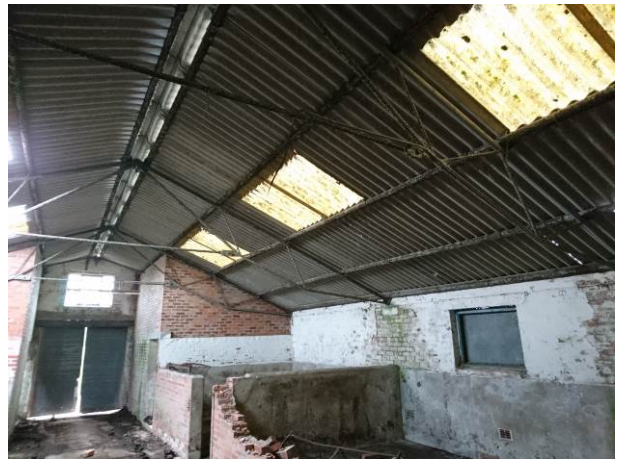
Roof over cow shed outrigger.
