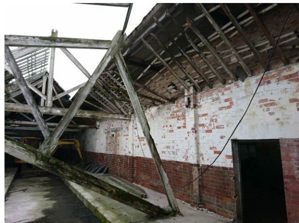
Collapsed truss supporting roof.
