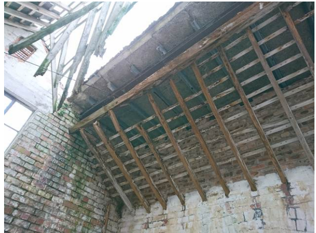
Partial collapse of roof over outrigger.
