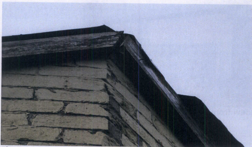
Figure 4.4 Barge boards with gaps beneath
