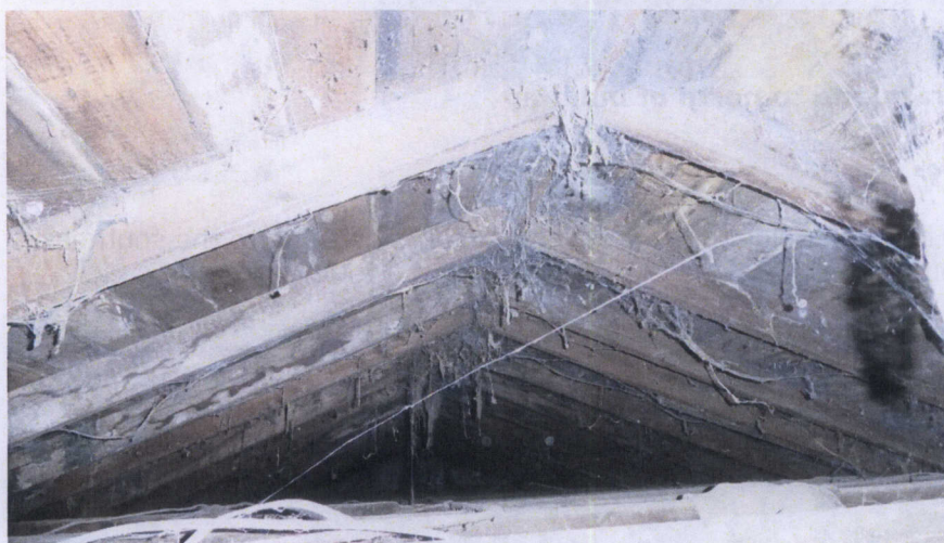
Figure 4.6 Cobwebs in loft space
