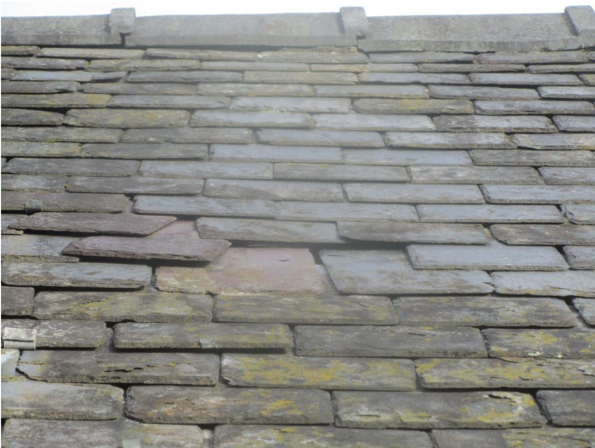
Image 12 Slipped roof tiles on B2
