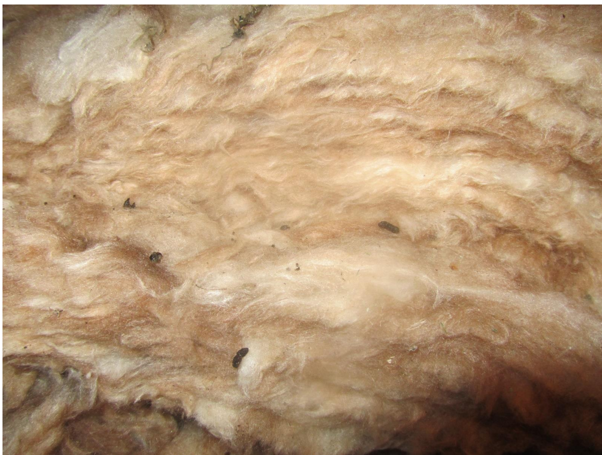
Image 14 Bat droppings found on the floor near to the hatch within the loft void of B2
