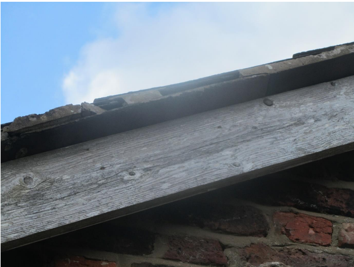
Image 6 Mortar gaps on the western gable end of B1
