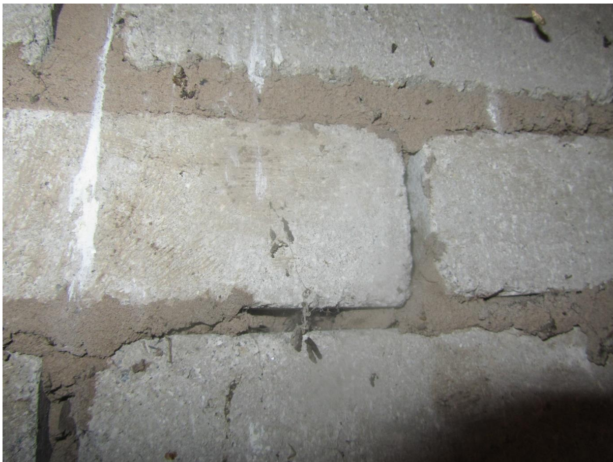
Image 13 Bat droppings stuck to the internal northern gable wall inside the loft void of B2 (also showing bird droppings)
