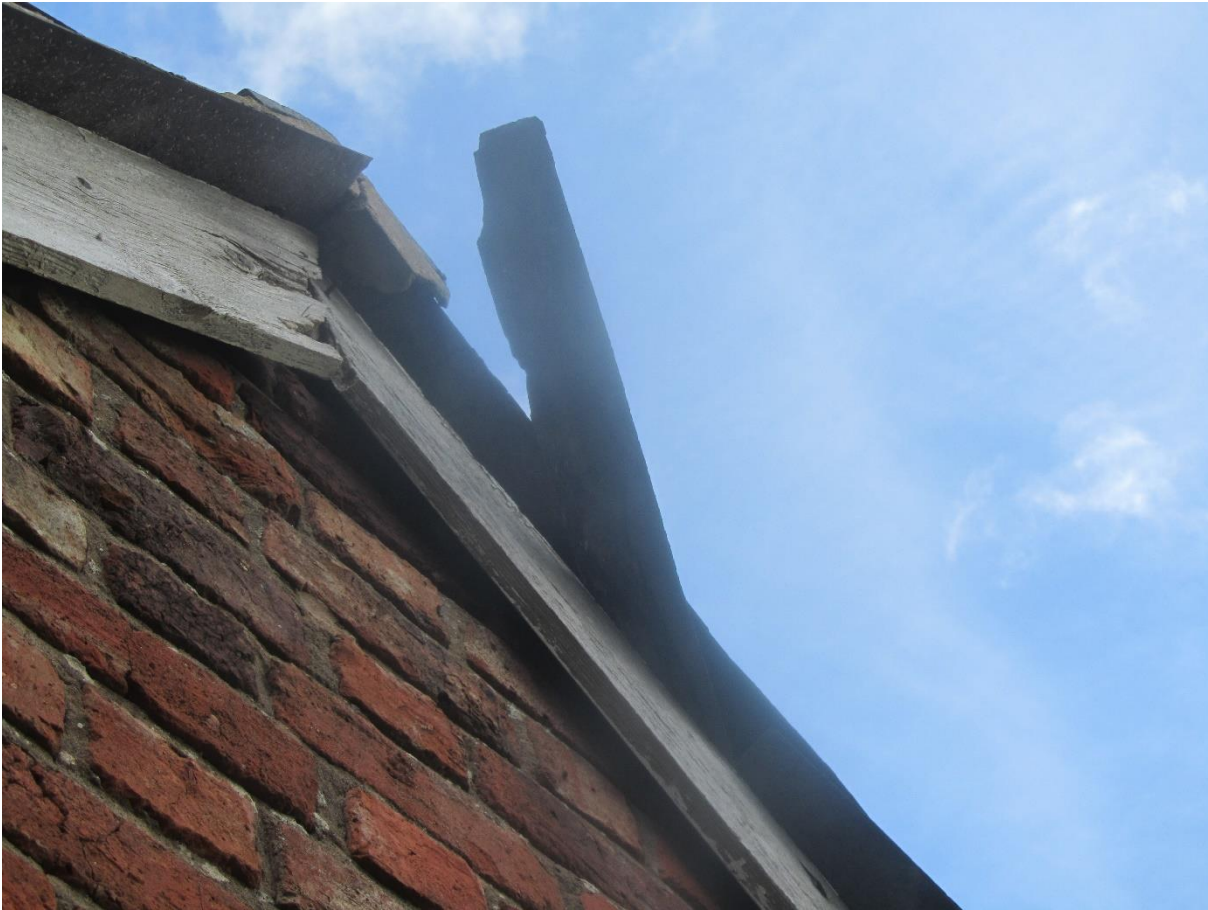
Image 11 Damaged roof at the southern gable end of B2
