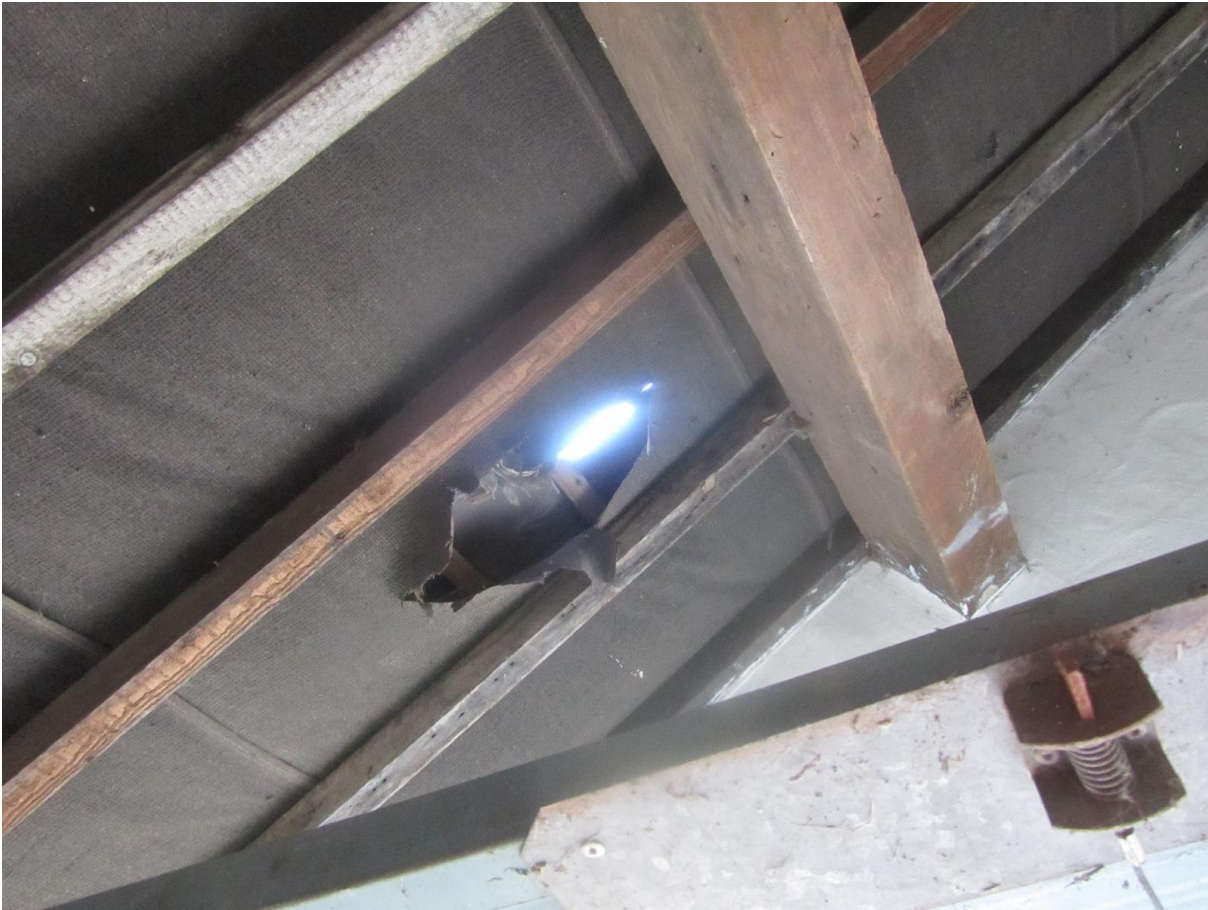
Image 7 Tear in the roof lining and tile gap, viewed from inside B1
