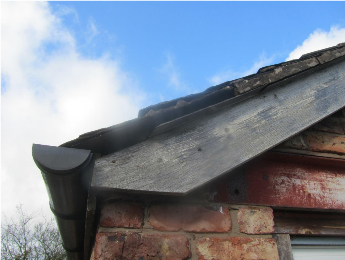
Image 5 Mortar gap on the eastern gable end of B1
