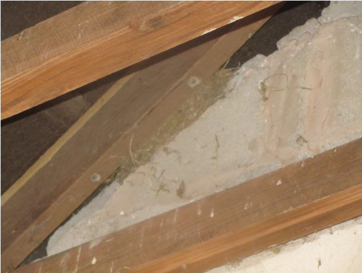
Image 25 Disused passerine bird nesting found inside a stable block section of B3
