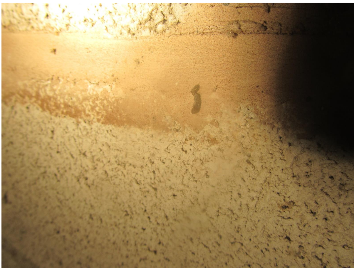
Image 24 Bat droppings found on the wall below crevices between the timbers and internal eastern gable wall inside the barn section of B3
