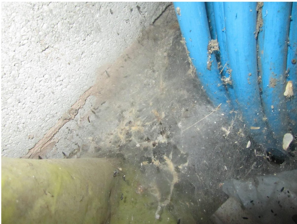
Image 23 Accumulation of bat droppings found inside eastern-most table block section of B3, on the wall and stuck in cobwebs
