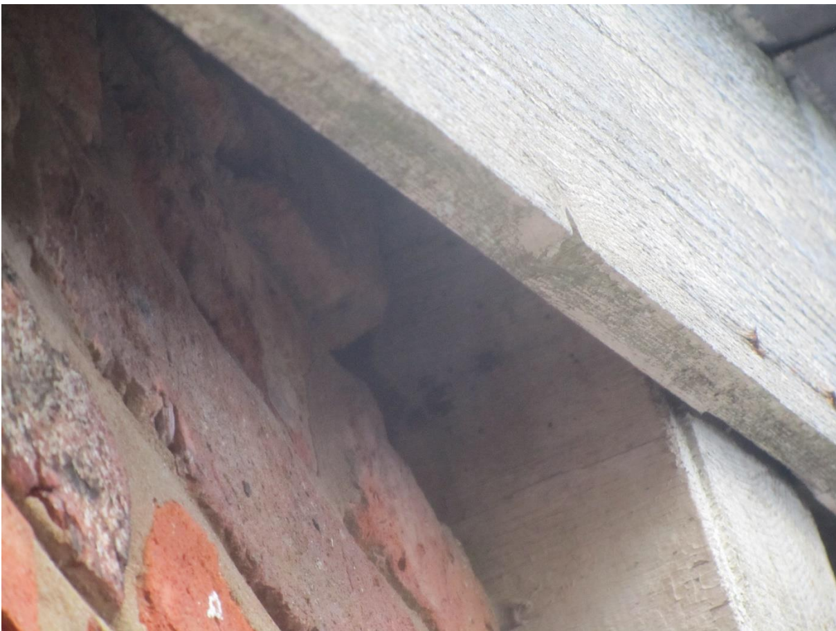
Image 8 Small gap between the timbers and external wall on the eastern gable end of B1
