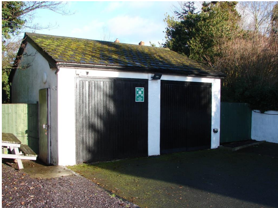
View of Side D with Side C on the left of the view. The hole in the barge board is at the corner of Side C and Side D.
