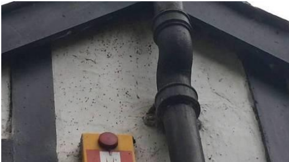
Close up of droppings at north elevation
