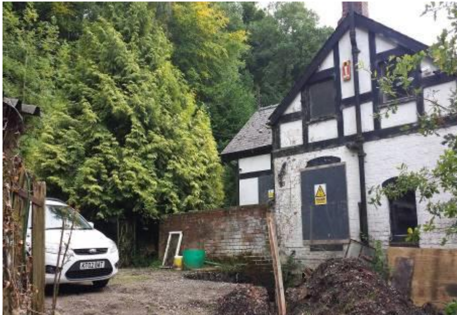
Location of droppings on the north elevation exterior render
