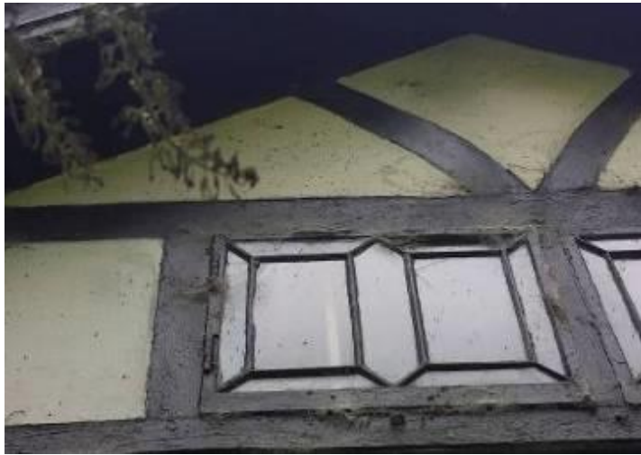
Droppings on the east facing elevation
