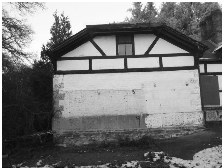
Southern elevation showing weathering, paint discolouration and previous work marks
