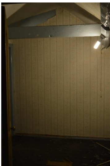
Low light level in first floor landing
