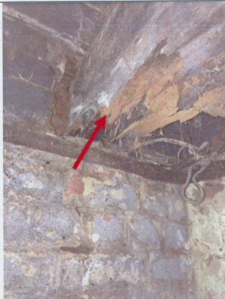
Fig 7- significant timber decay
