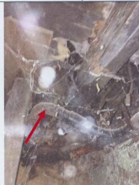
Fig 12- decayed floorboarding and joists
