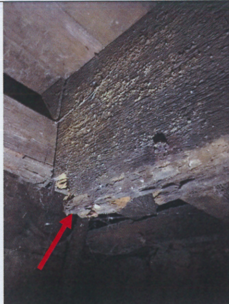
Fig 1- significant timber decay- joist
