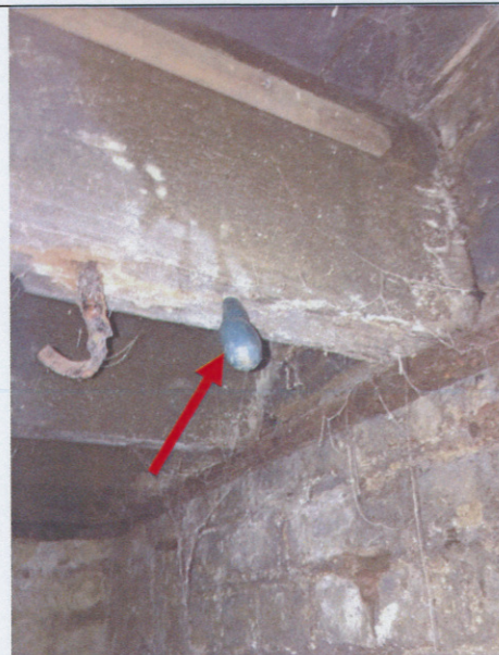
Fig 9- significant timber decay-embedded probe
