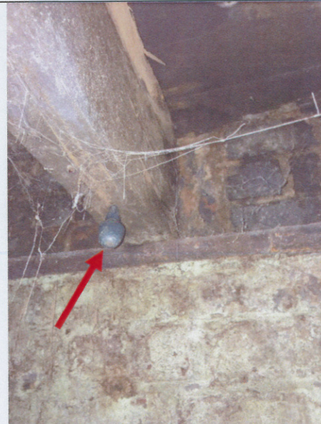
Fig 10- significant timber decay- joist-embedded probe
