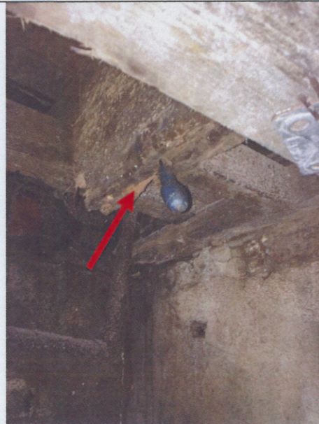
Fig 6- significant timber decay- joist- embedded probe
