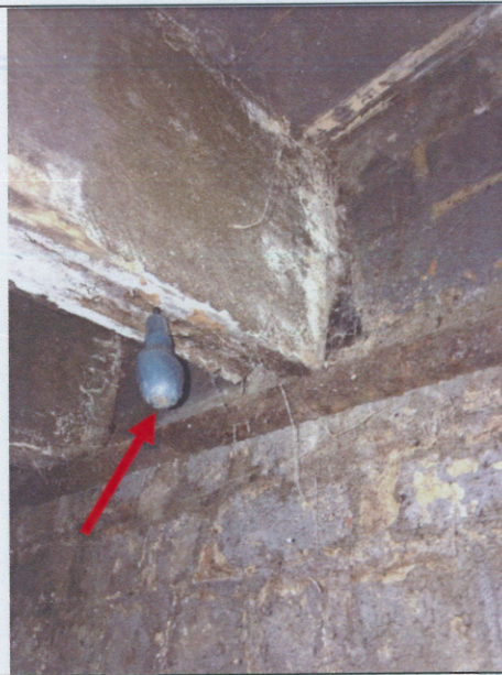
Fig 8- significant timber decay- joist-embedded probe
