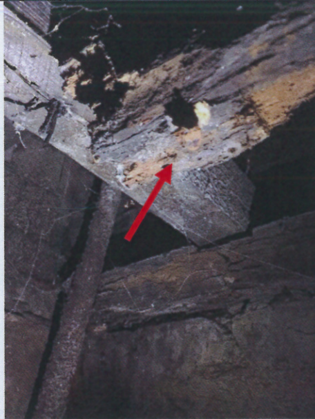
Fig 2- significant timber decay- joist
