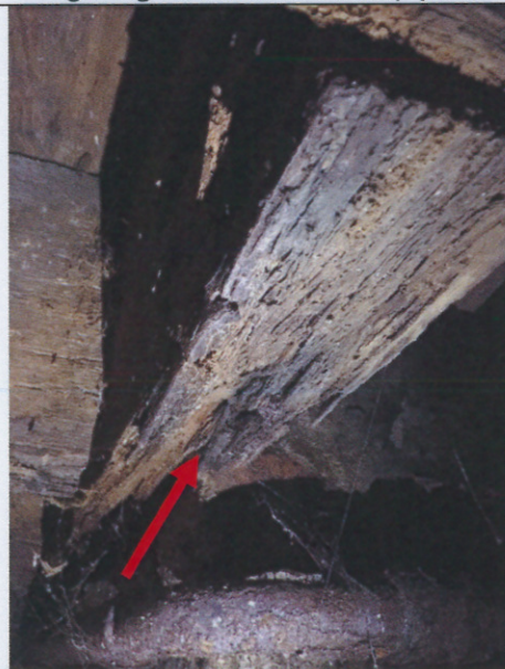
Fig 3- significant timber decay- joist
