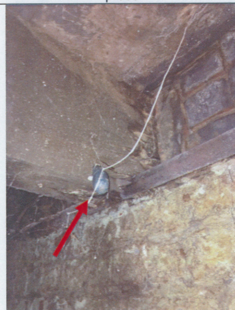
Fig 11- significant timber decay-embedded probe
