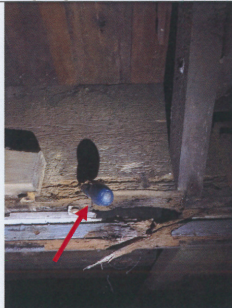
Fig 5- significant timber decay- joist- embedded probe
