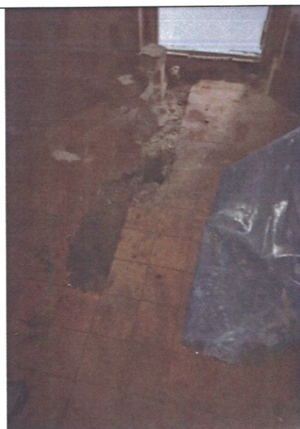
Fig 14- water ingress- tiled floor
