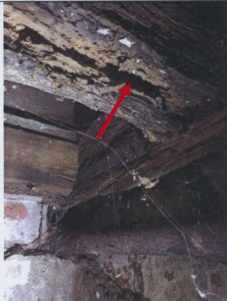
Fig 4- significant timber decay- joist
