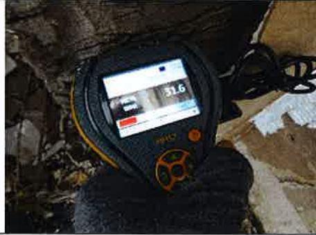
Fig 4- elevated moisture meter readings
