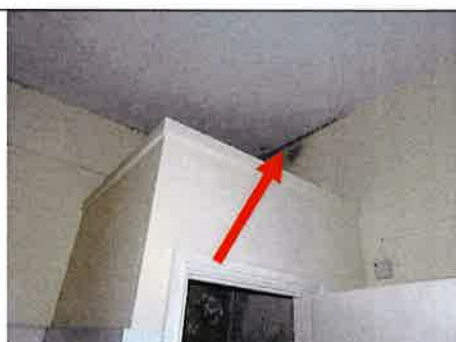
Fig 10- junction between walls
