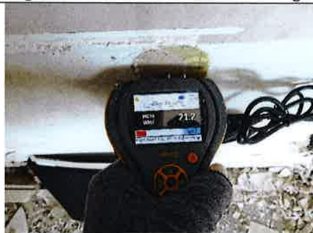
Fig 6- elevated moisture meter readings
