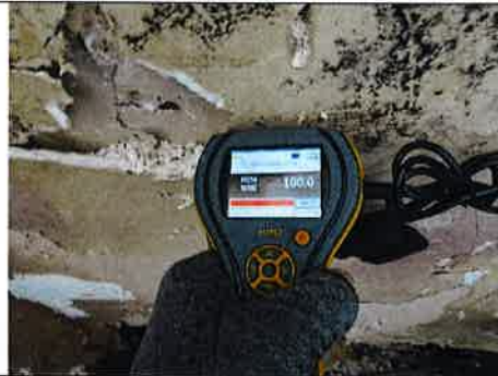
Fig 2- elevated moisture meter readings
