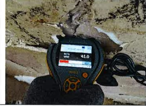
Fig 3- elevated moisture meter readings
