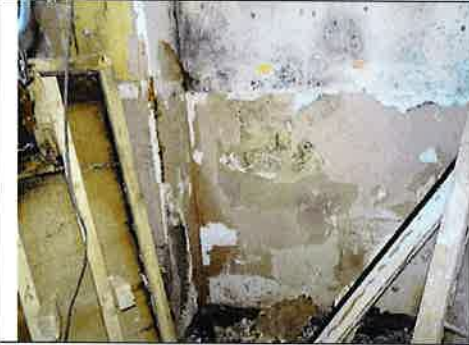
Fig 1- detached and degraded drylining
