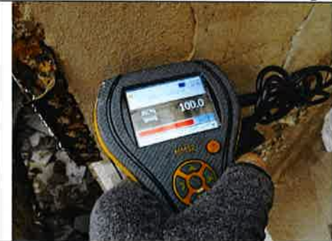
Fig 5- elevated moisture meter readings
