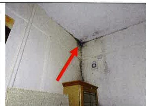
Fig 9- junction between walls
