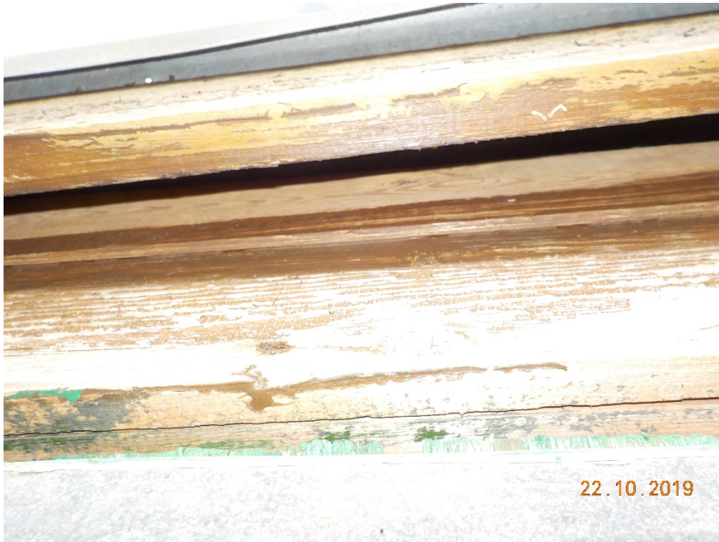
Plate 9: View of gap between fascia boards on Building 1
