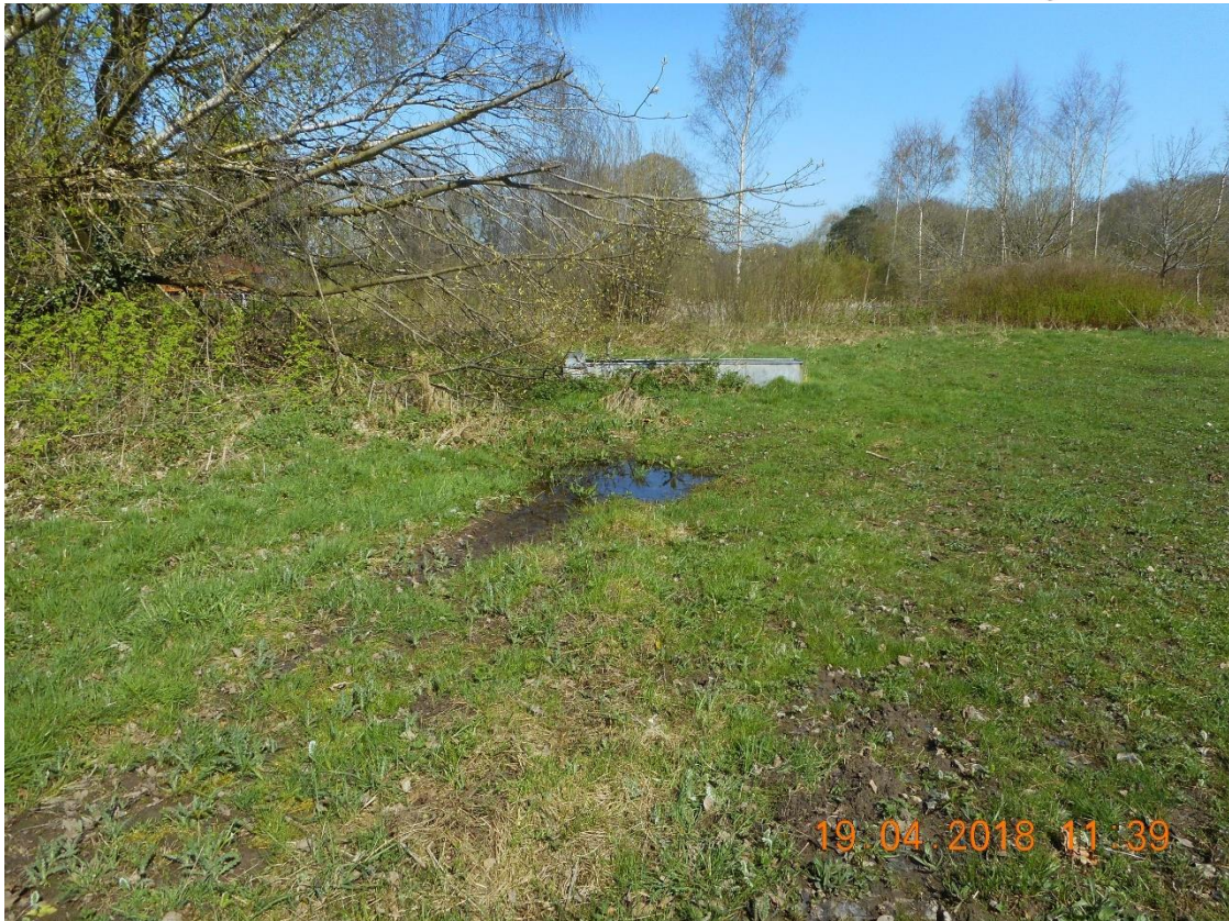
Figure 3: Waterlogged ground on site
