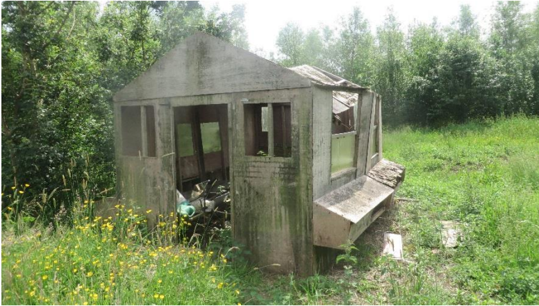
Image 3.11 Dilapidated chicken coups to the west of the site (B1 & B2)
