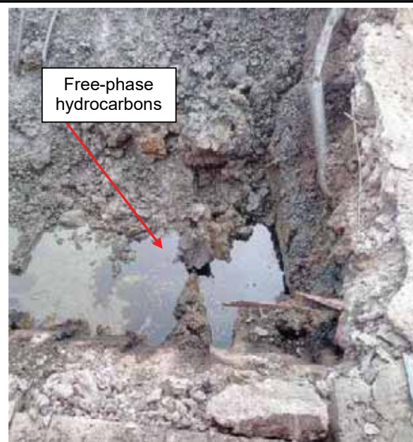
Photograph Four - TP101 - free-phase hydrocarbons, suspected fuel line source.
