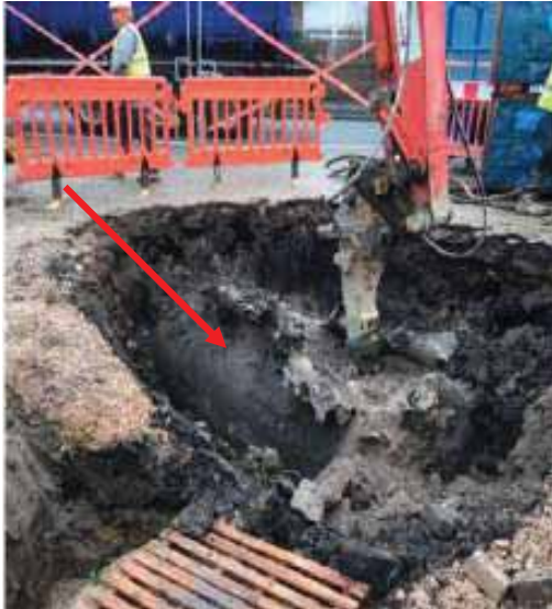
Photograph Twenty-Six - Third abandoned tank found adjacent to the old interceptor. Concrete slurry filled.
