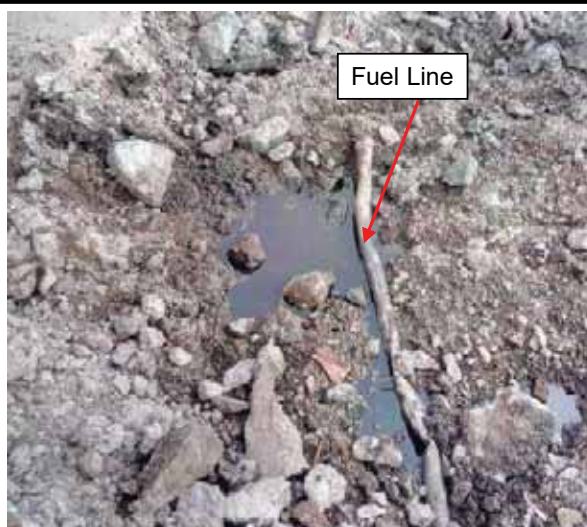
Photograph Two - Old fuel lines in a pool of hydrocarbon impacted water in TP102
