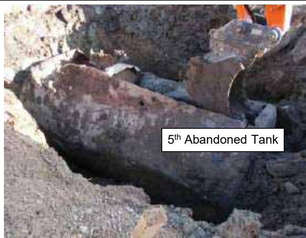
Photograph Thirty-Four - Abandoned Tank 5
