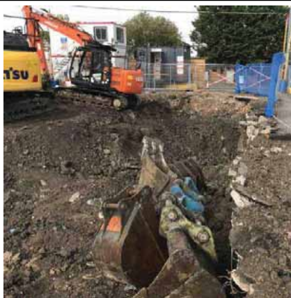
Photograph Eight - EX001 (Tank farm) looking north.
